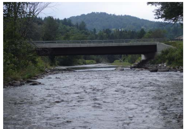
Figure 21: Looking upstream towards Route 114 Bridge on Reach T102B, Riverside Center on left. Sediment deposits and channel widening evident.
