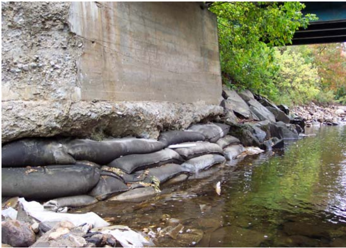
Figure 16: View looking upstream beneath Burrington Bridge (in background) and the covered bridge on Reach T102A taken in 2003. Channel degradation evident with reinforcements necessary beneath original footings. Stream level was formerly at base of concrete footing.
