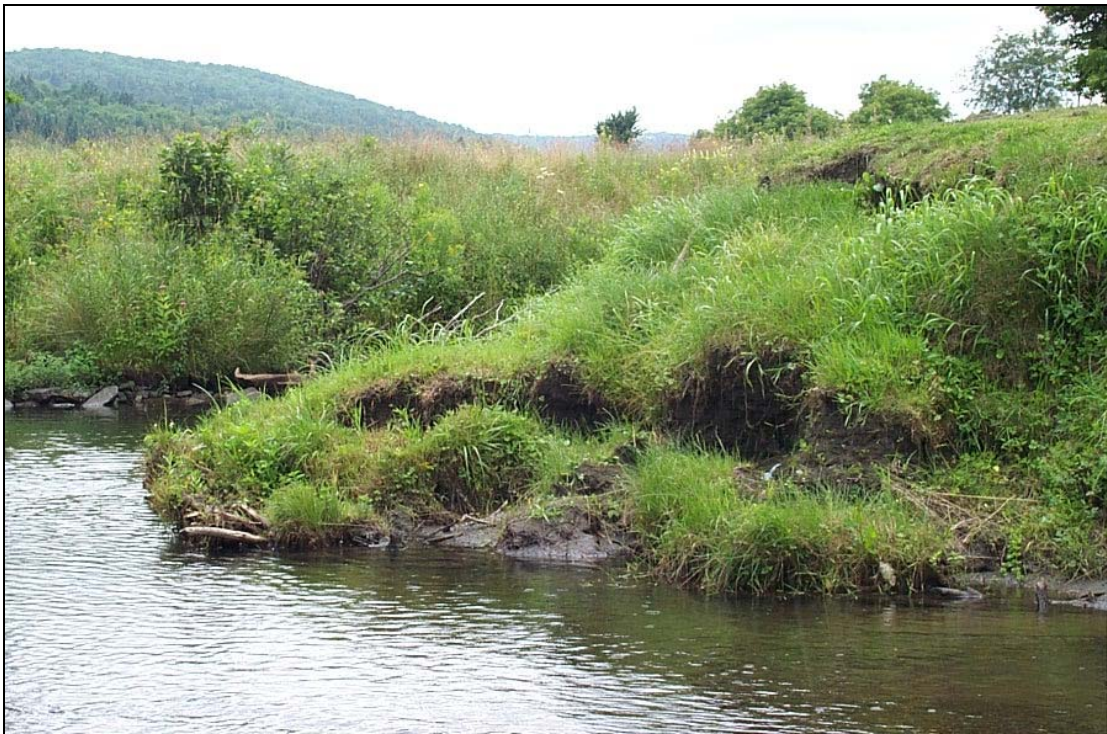
Figure 3. Bank erosion in segment M02-B adjacent to Durant cemetery. The Cabot Cemetery Commission stabilized approximately 300 linear feet of bank with rock riprap during fall 2004.
