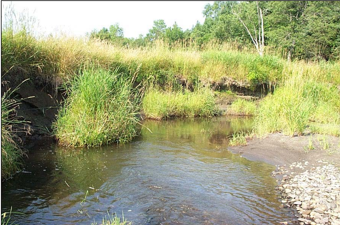
Figure 14. Segment M05-B was noted to have extensive lateral bank erosion on the outside bends.
