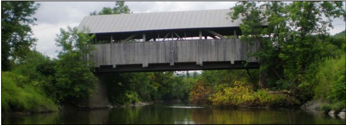
Figure 12: The Coburn Covered bridge (R24) was elevated to increase the area through which water can flow. Despite this, the bridge abutments still constrict the channel and upstream and downstream erosion is a result (see fallen tree on right bank).
