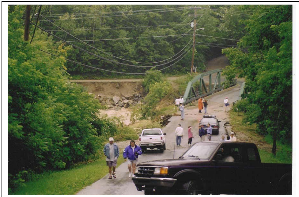
Photo 10. (M14) South Street Bridge approaches eroded, 1998 flood. K. Underwood collection.
