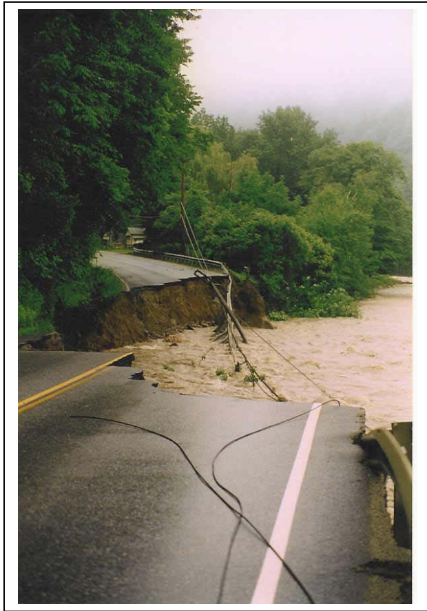
Photo 9. (M15) Route 116 washout, 1998 flood. K. Underwood collection.
