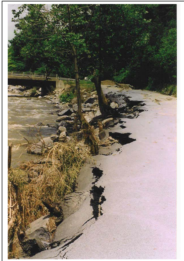
Photo 12. Hewitt Road Bridge outflanked and Notch Road washed out, 1998 flood. K. Underwood collection.
