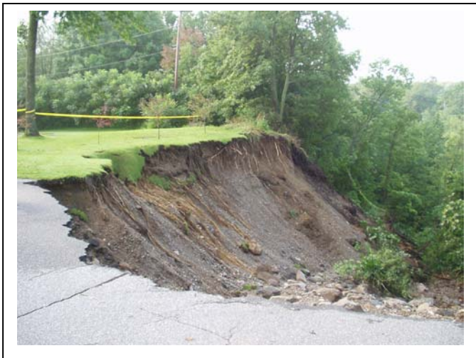
Figure 9. Slope failure behind (southwest) of Merchants Bank along West Street (Route 17 / 116) in Bristol, 28 August 2004.
