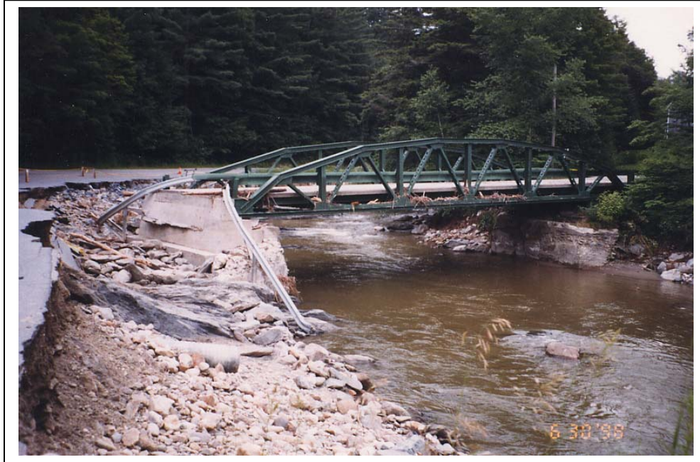
Photo 3. (M17) York Hill Road Bridge, approaches washed out, 1998 flood. View from west. Susan Tucker collection.
