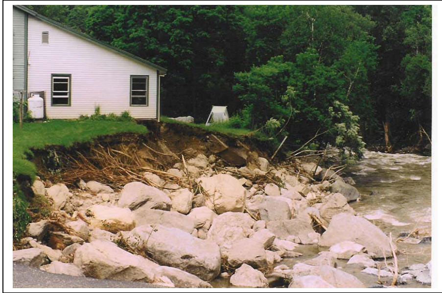
Photo 11. Streambank erosion and undermining of residence, immediately downstream of South Street Bridge, 1998 flood. K. Underwood collection.
