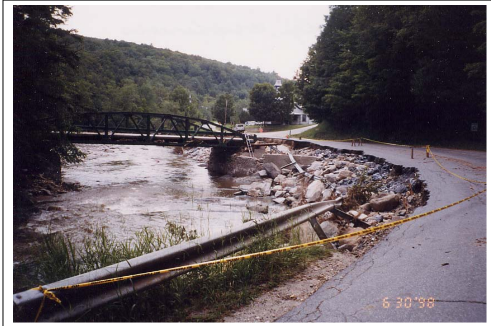
Photo 5. (M17) York Hill Road Bridge, approaches washed out in 1976 flood. View from east. Addison Independent, 1976.
