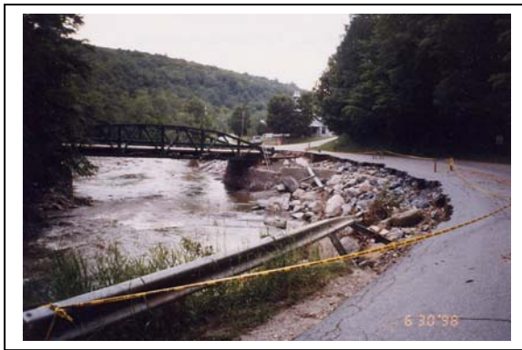
Figure 1. York Hill Bridge, West Lincoln, following June 1998 flood. (Photo Credit: Susan Tucker)
