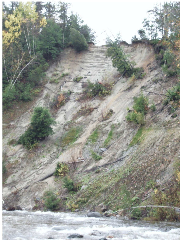
Figure 1. Mass failure or landslide on west bank of Reach M25, looking upstream from east shore.
