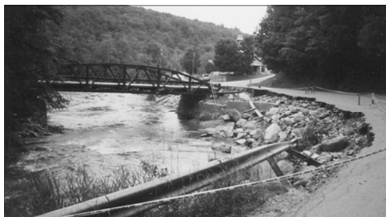
York Hill Bridge, West Lincoln, following June 1998 flood. Photo Susan Tucker
