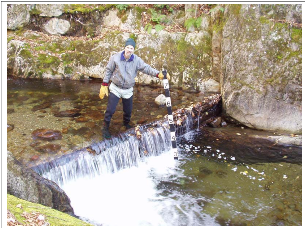
Photo 1. Dam across Middle Branch (Reach M14) in approximate location of D.C. Sherman mill dam noted on 1871 Beers Atlas of Ripton, VT. (Warren King pictured)
