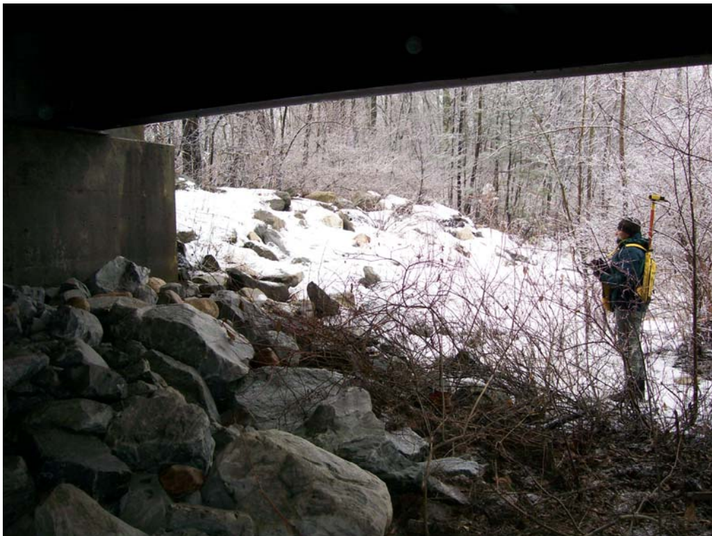
Figure F-4: Under Route 7A Bridge from left sidebar looking toward upper left berm.
