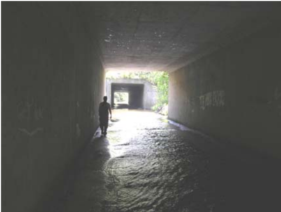
Figure 40. Route 4 highway box culvert crossing structures. View downstream; foreground is box culvert under exit ramp approximately 90 feet long; background is culvert under Route 4 east-bound and west-bound lanes, approximately 220 feet long.
