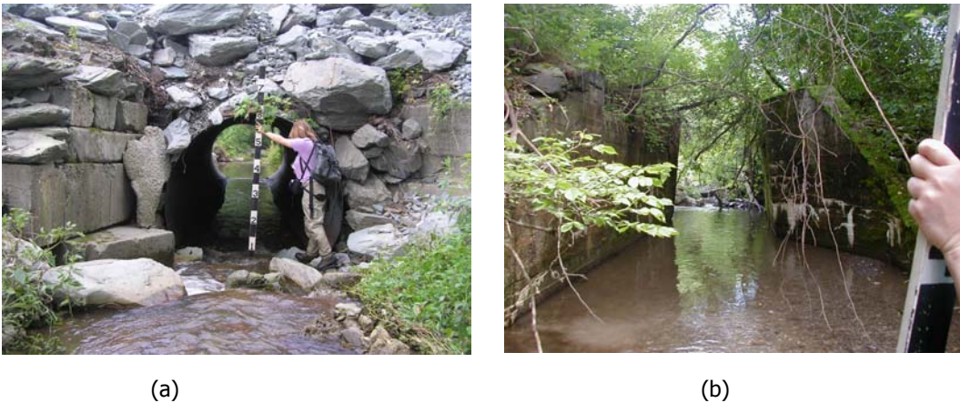
Figure 55. Constriction along reach T02.08-s1.02 of Pond Hill Brook. (a) Culvert crossing for driveway to Hadeka Stone Corporation off Staso Road; view downstream to the culvert inlet. (b) Old abutments approximately 300 feet downstream from culvert crossing; view downstream.
