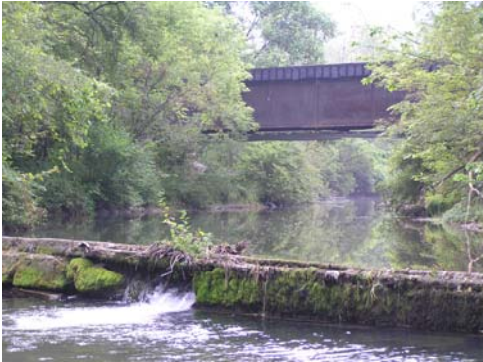
Figure 12. Low-head dam in reach T02.09, located just downstream of the confluence of North Bretton Brook, approximately 350 feet downstream of the Route 4A crossing, and 110 feet downstream of the railroad crossing. (View upstream on 11 August 2005).
