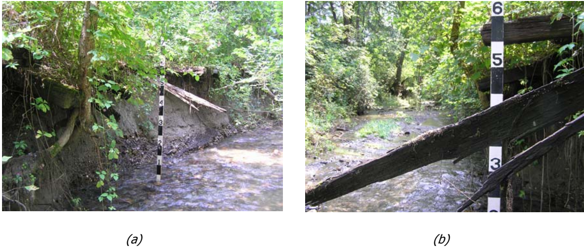
Figure 58. Pond Hill Brook is regaining sinuosity and building new floodplain through by actively eroding the bed of the abandoned railroad spur leading to the former Staso Milling Company (Segment E of reach T02.08-s1.01). (a) view downstream to left bank; (b) view upstream from left bank, railroad ties are undermined and collapsing into the channel. Viewed 31 July 2006.
