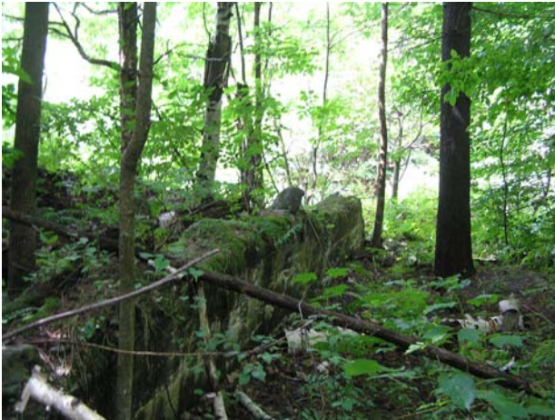
Figure 26. T02.11-s1.04-A. Remnants of vertical concrete wall / dam at former reservoir site located mid-segment. View (to the southwest) from right bank corridor toward the channel and mill pond.
