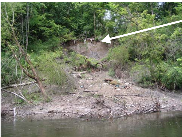
Figure 22. High bank erosion along the right bank of the Castleton River is exposing household rubbish in the former Fair Haven landfill.
