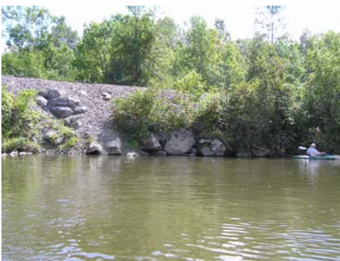
Figure 14. Length of armorment on left bank (view facing downstream) along the Clarendon-Pittsford railroad, reach T02.04.
