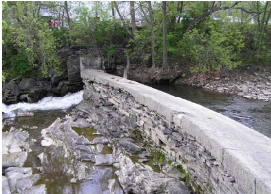
Figure 17a. Dam 2 – Structural Slate Dam, view to north from southern end of dam. Breach evident at north end. 18 May 2005, during moderate to low flows.
