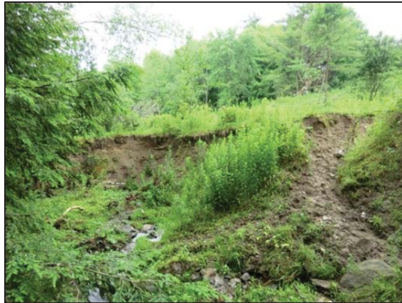
Figure 5.23. Severe bank erosion was documented along both banks in M04S1.02-B.
