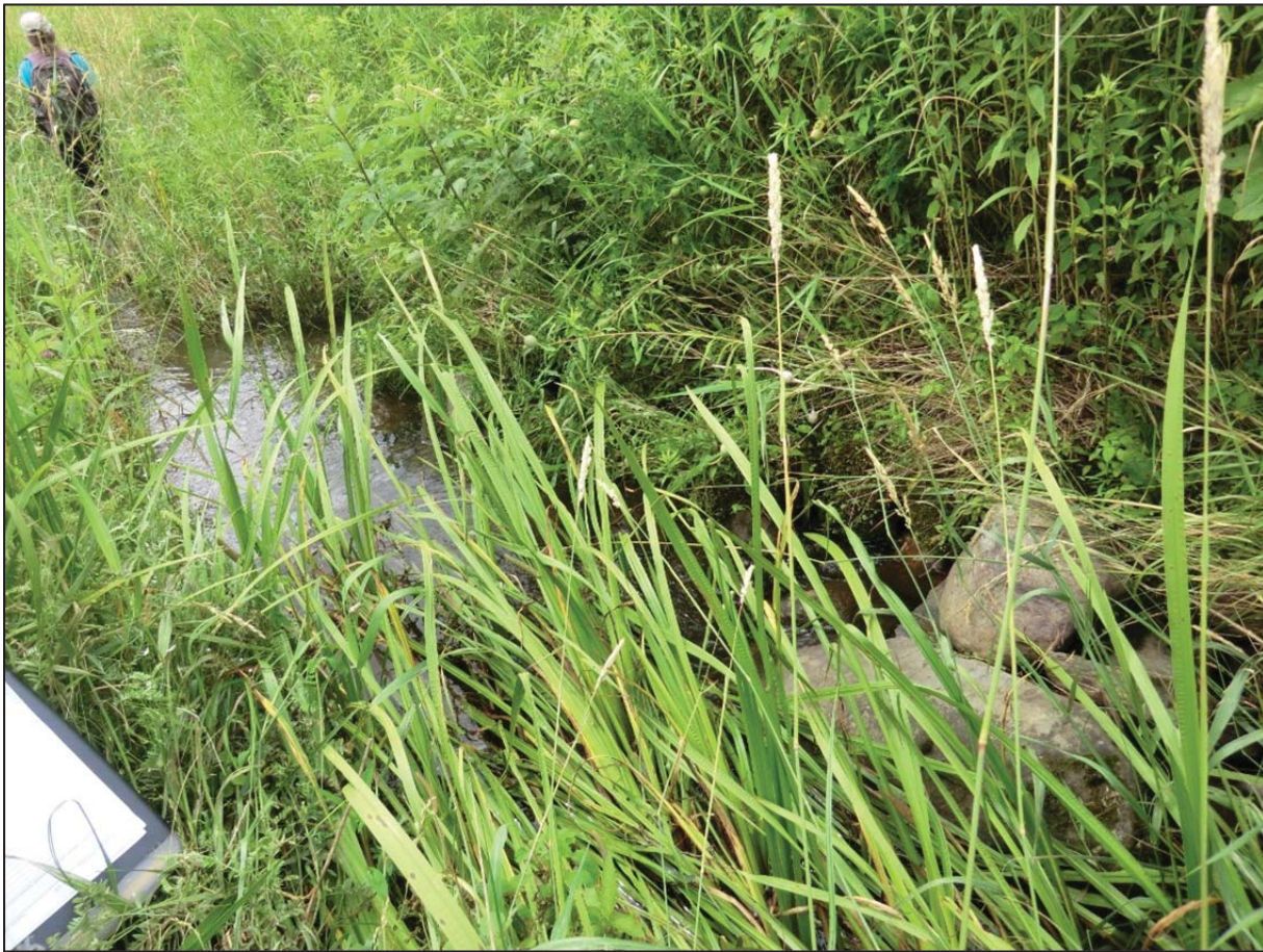
Figure 5.33. Old riprap in the channel in M06S2.02-C.
