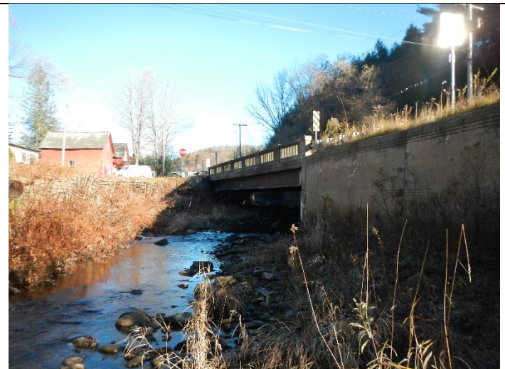
Incised channel at the intersection of Route 112 and Holbrook Road.
