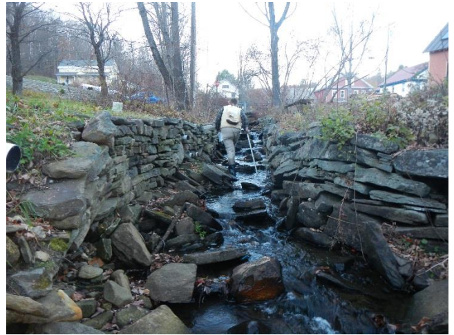
Figure 4.11: Extreme bank armoring on segment M07.A.
