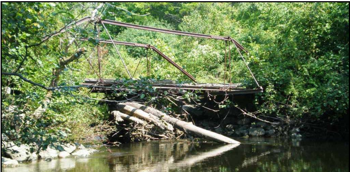
Figure 11: The abandoned bridge (M29) is similar to several nearly abandoned crossings that are likely to cause debris and ice jams and may washout and cause further damage in a future flood.
