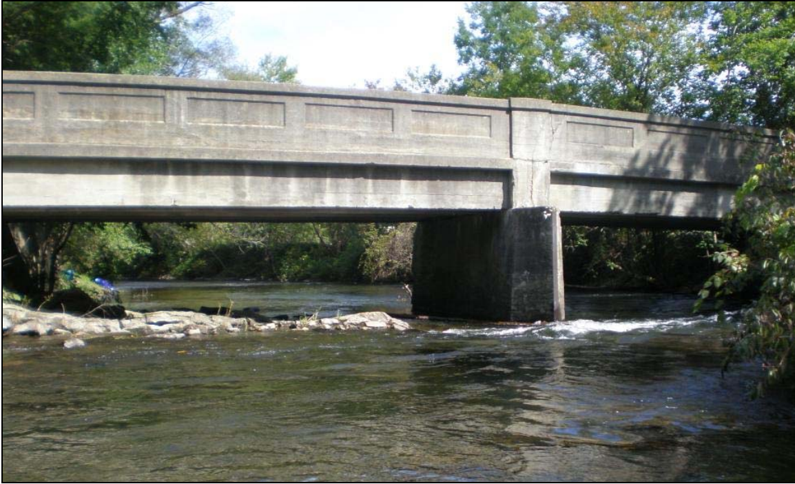
Figure 9. Bedrock and a pier block flow at the Creek Road Bridge on M27.
