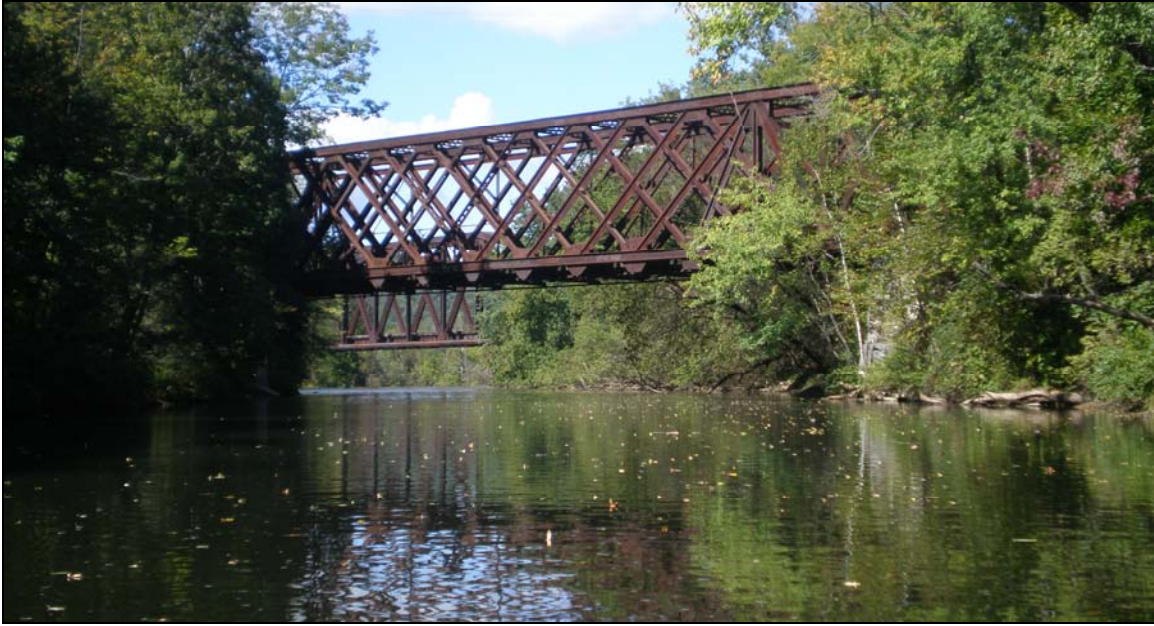
Figure 14. Dual railroad bridge crossings upstream of the Mead Falls and Omya dam which create a backwatered segment with a very low water surface slope.
