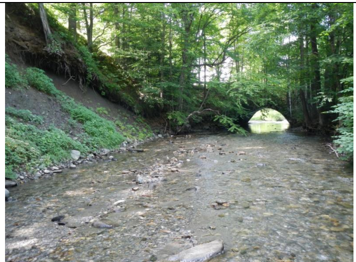
Undersized arch and downstream mass failure
