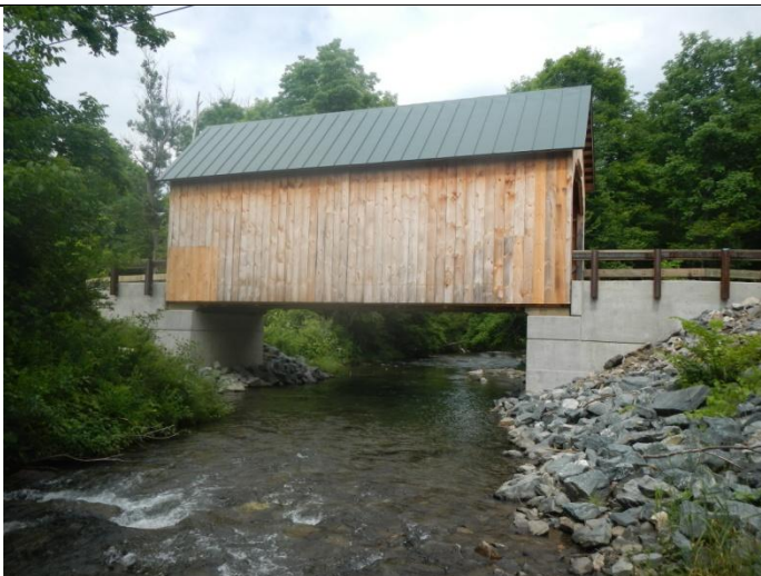
Major constriction at the Bible Hill Rd bridge
