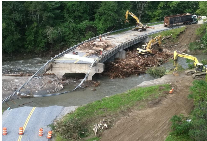
Figure 5.1: Tropical Storm Irene damage to the Route 44 bridge over Mill Brook in reach M04 (photo from www.windsorvt.org ).
