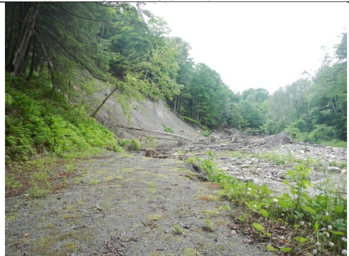
Major widening, mass failure, and Brook Road washout
