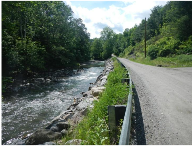
Figure 4.10: Extensive bank armoring along Brook Road on segment M05.C.
