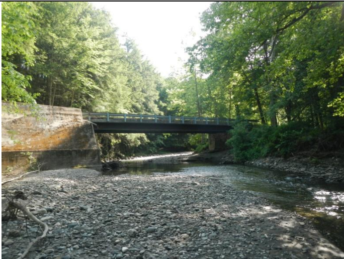
Aggradation at the lower Brook Rd bridge
