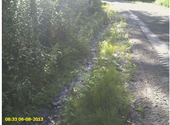
Figure 19: Unstable ditch #2 west of intersection with Robtoy Road (photo by LCPC)
