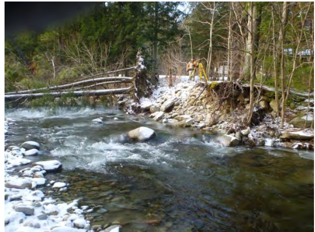
Figure 2: Major bank erosion towards the well head and undermining of large trees.
