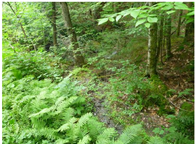
Figure 21: Outlet of an 18" culvert to the north side of Canyon Road just west of waterfall.
