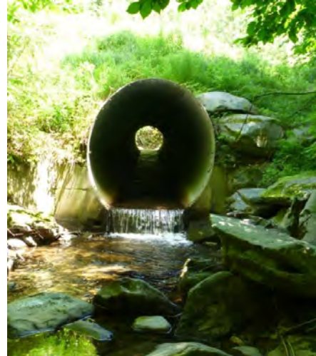
Figure 14: Perched culvert beneath lower Canyon Road
