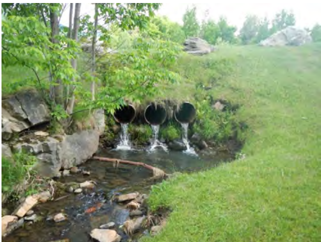
Figure 16: Three culverts at the outlet of the trout pond created by a small dam on reach T7S1.01.
