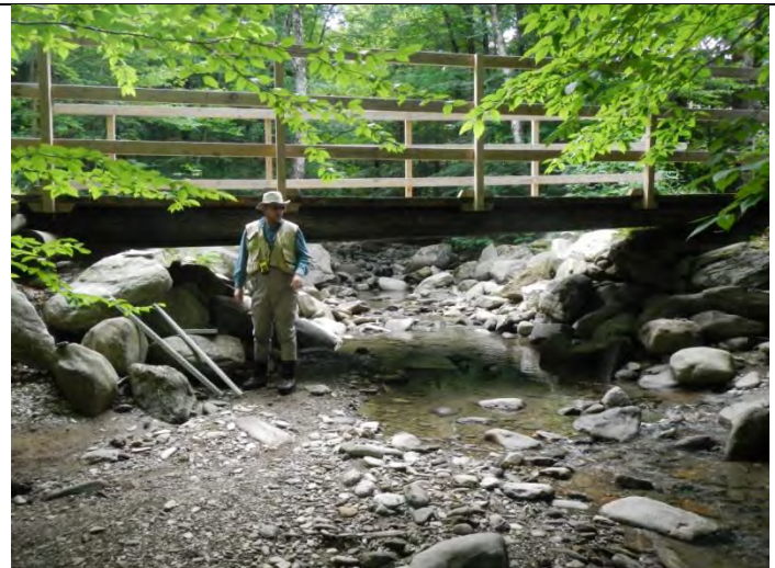
Major constriction from bridge abutments at upper footbridge
