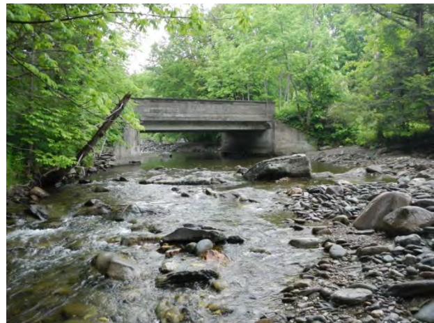
Figure 8: Bankfull constriction and downstream deposition
