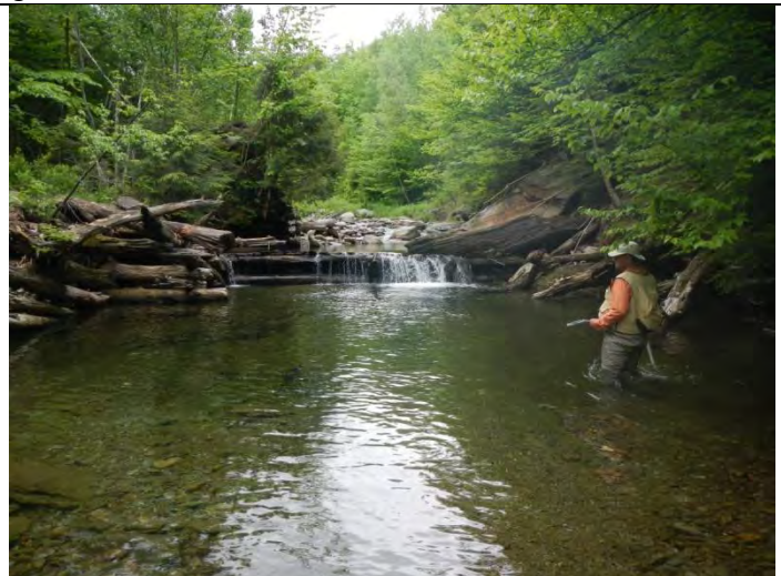
Failing timber crib dam, top of reach
