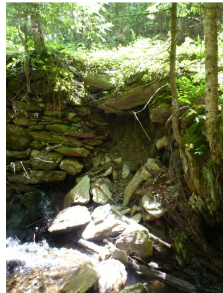
Figure 15: Failing stone wall embankment
