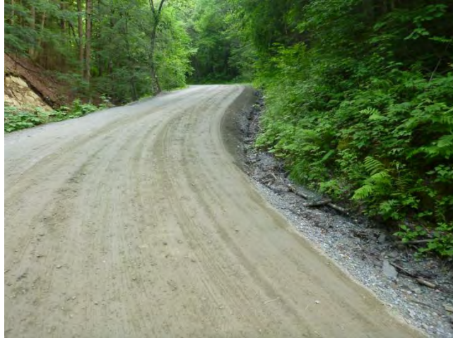
Figure 18: Unstable ditch #1 just uphill from first bend in Canyon Road
