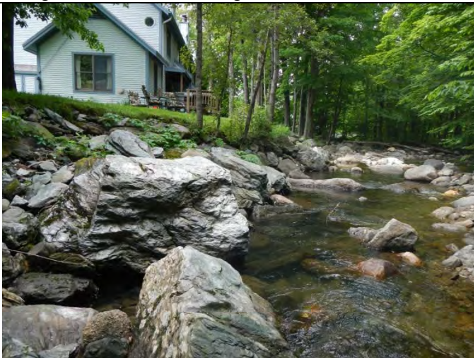
Development and incision with failing bank armor
