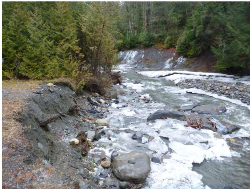
Figure 21: Bank erosion and mass failure on T3.09, Sleeper's River in Danville.
