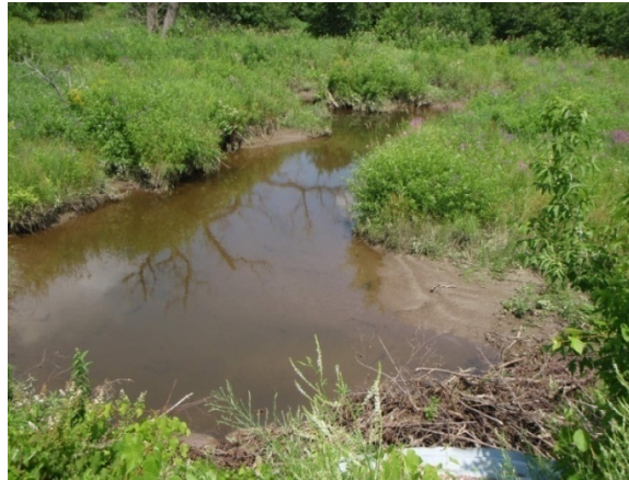
Figure 4.10 Looking upstream at the beaver dam impeding the inlet of the McMullen Rd culvert in reach M12
