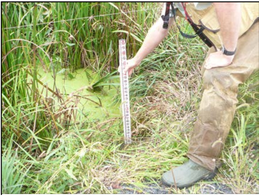
Figure 21. Undersized farm road culvert
