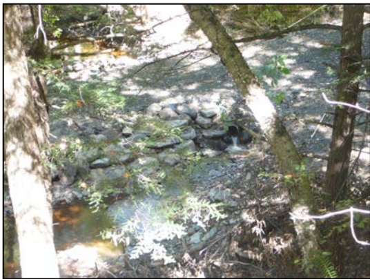
Figure 36. Private culvert with 12' freefall
