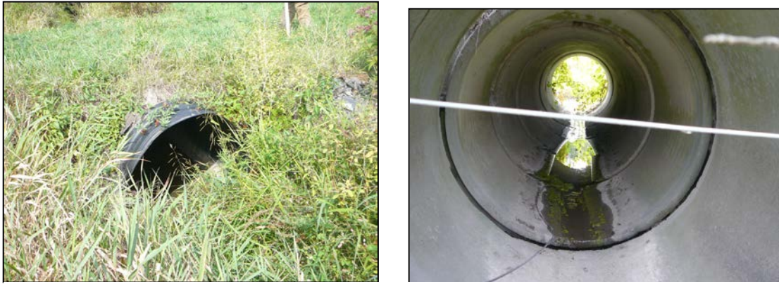
Figure 13. Undersized culverts for a farm road and Brown Lane
