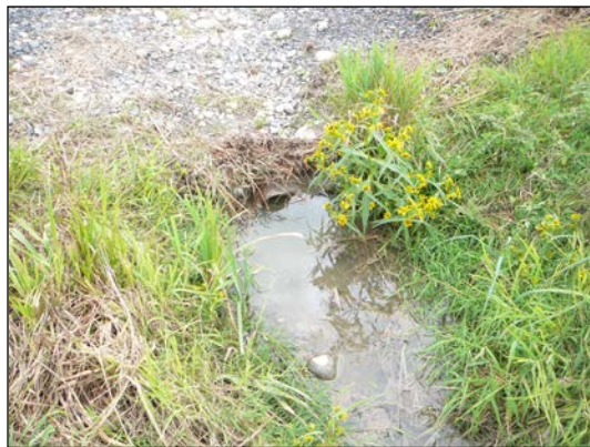
Figure 25. Undersized, squashed culvert
