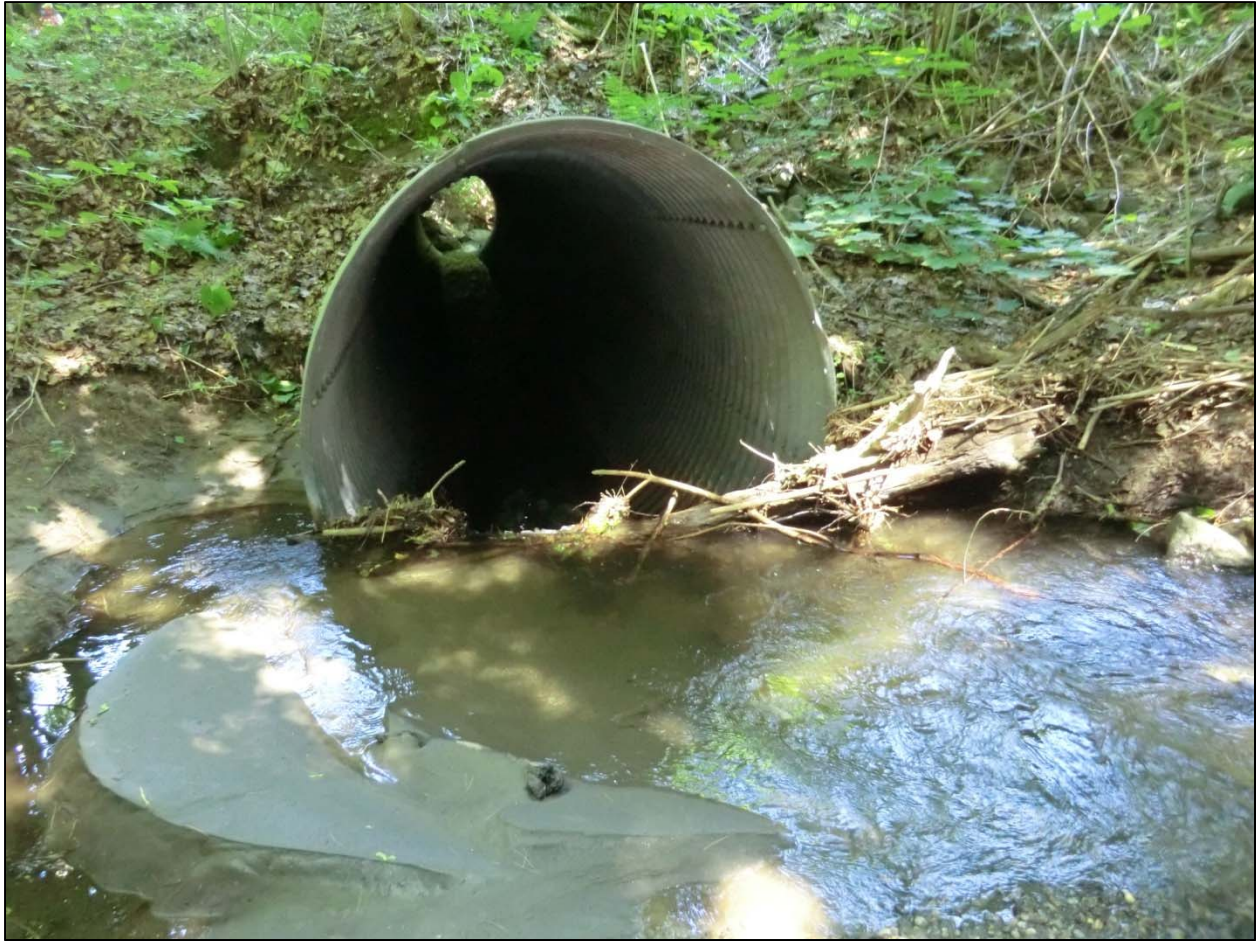
Figure 6.9. Undersized culvert on Valley St. is obstructed with sediment and debris (Project #6).
