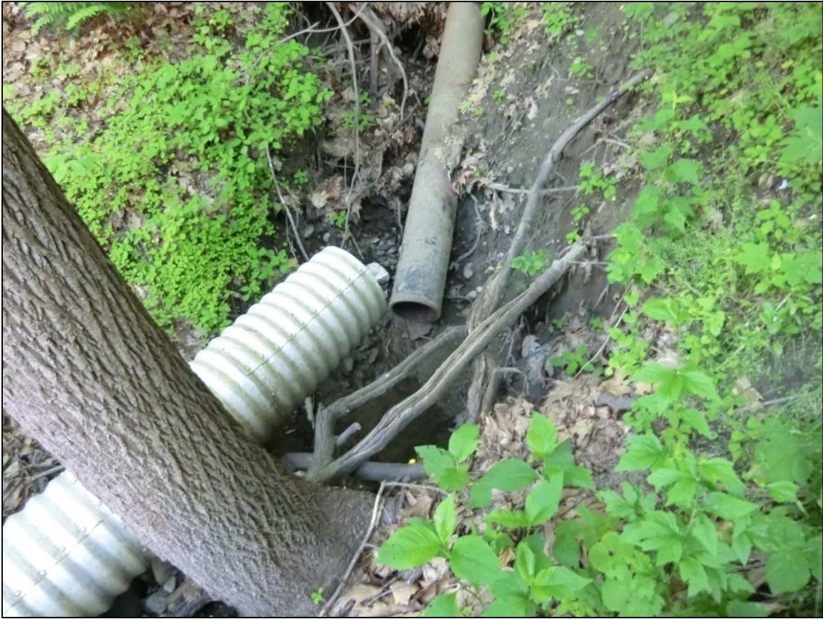
Figure 6.3. Broken pipe contributing to gully erosion off of Valley Street (see project #2).
