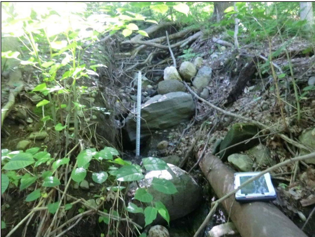
Figure 6.5. Gully erosion below broken off stormwater pipe (Project #3).
