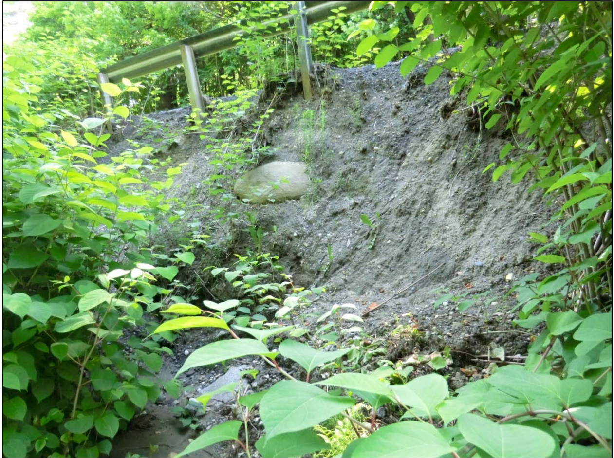
Figure 6.8. Potential washout location along Valley St. adjacent to study brook (Project #5).
