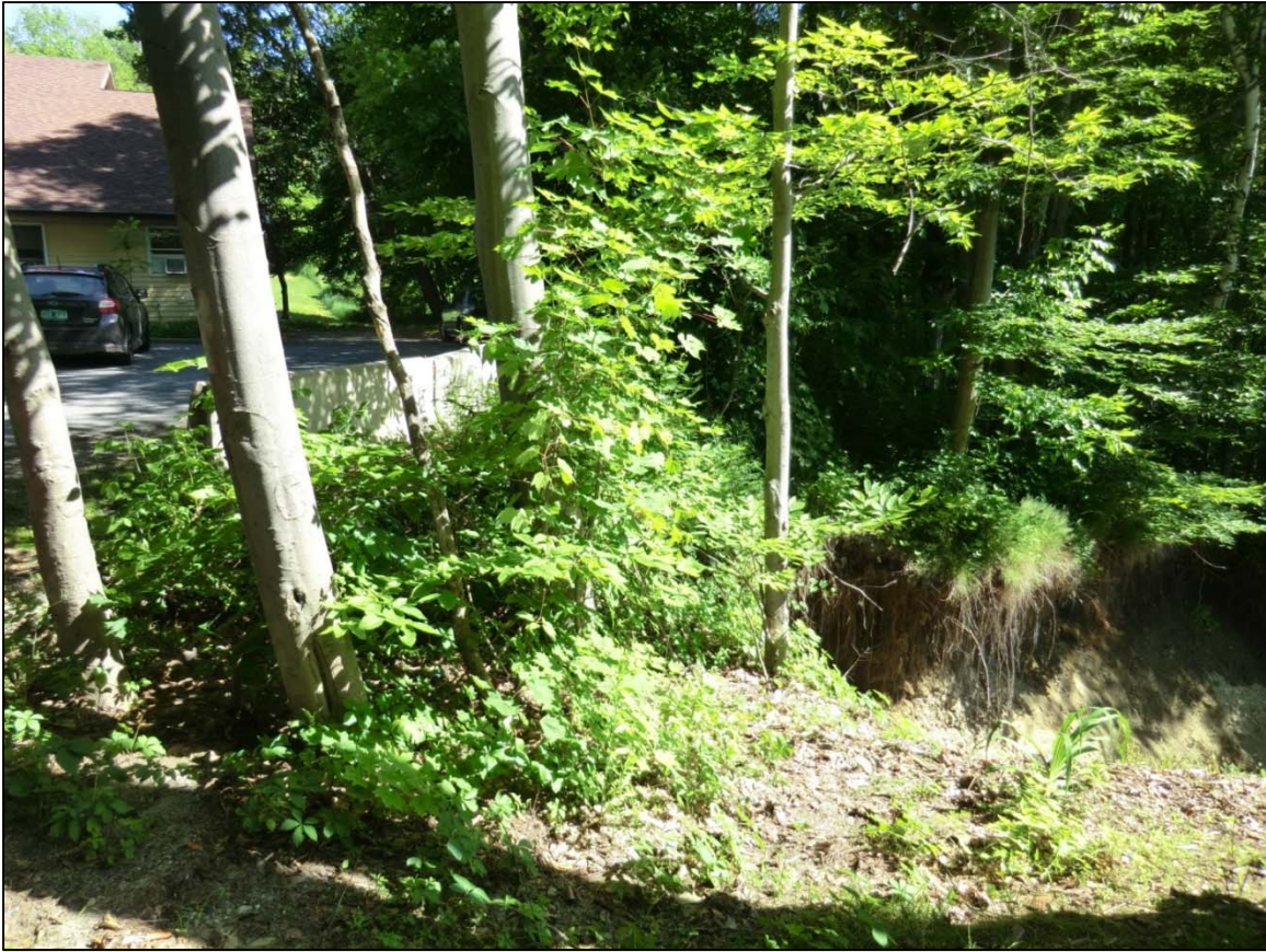
Figure 6.2. Severe erosion on valley wall near 10 Lincoln Street (Project #1).
