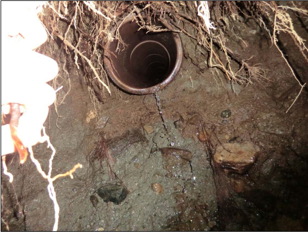
Figure 6.4 Broken stormwater pipe that is contributing to gully erosion (Project #3).
