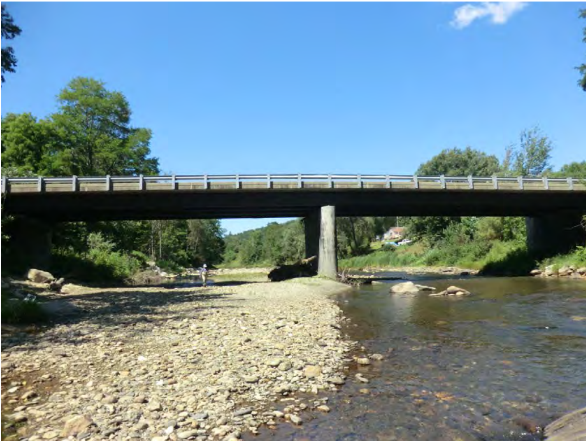
Figure 5.21. Bridgewater Village/Curtis Hollow Road Bridge causing upstream and downstream deposition in M22-A.
