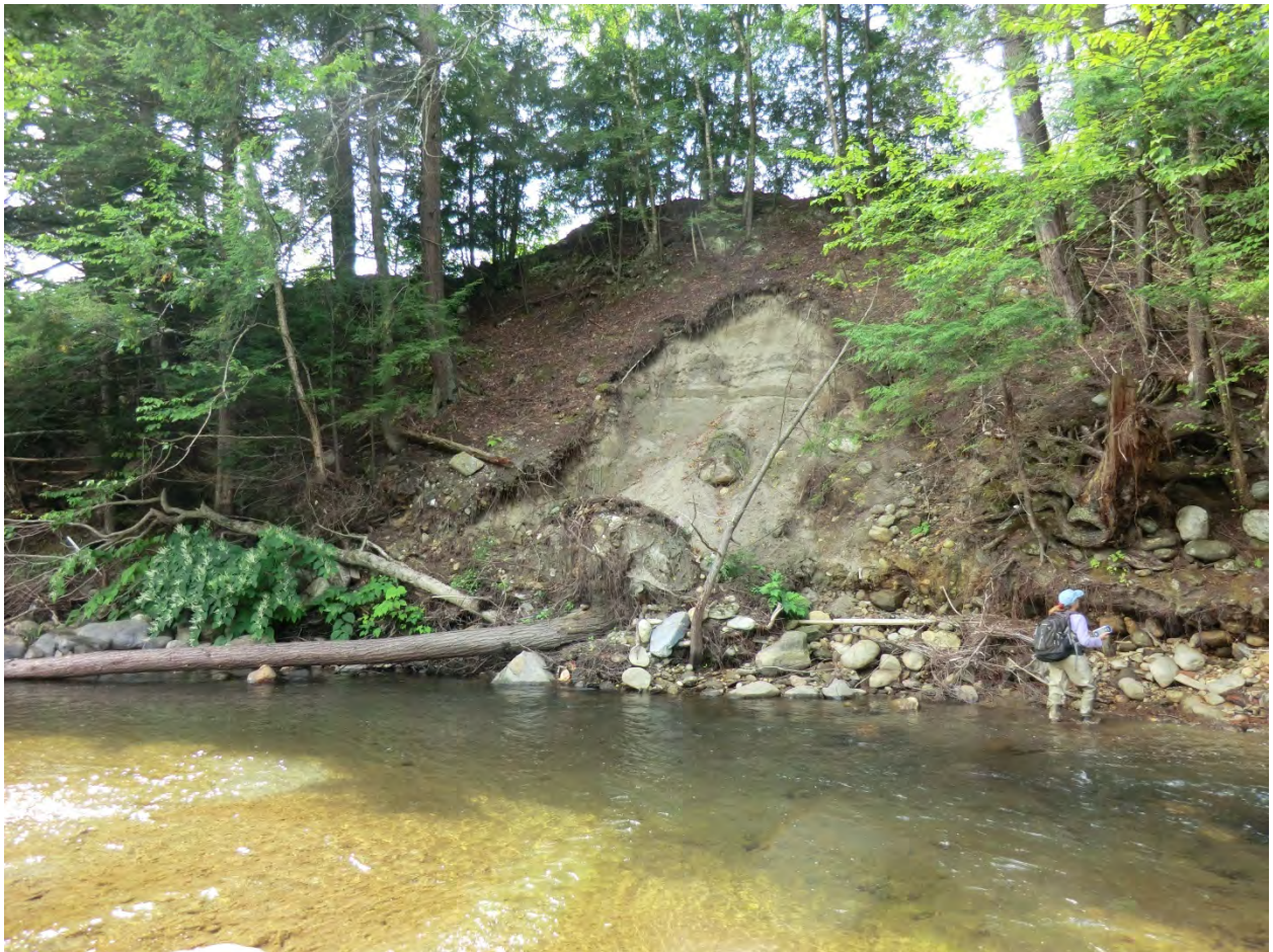
Figure 5.29. Mass failure on southern bank in M24-B.
