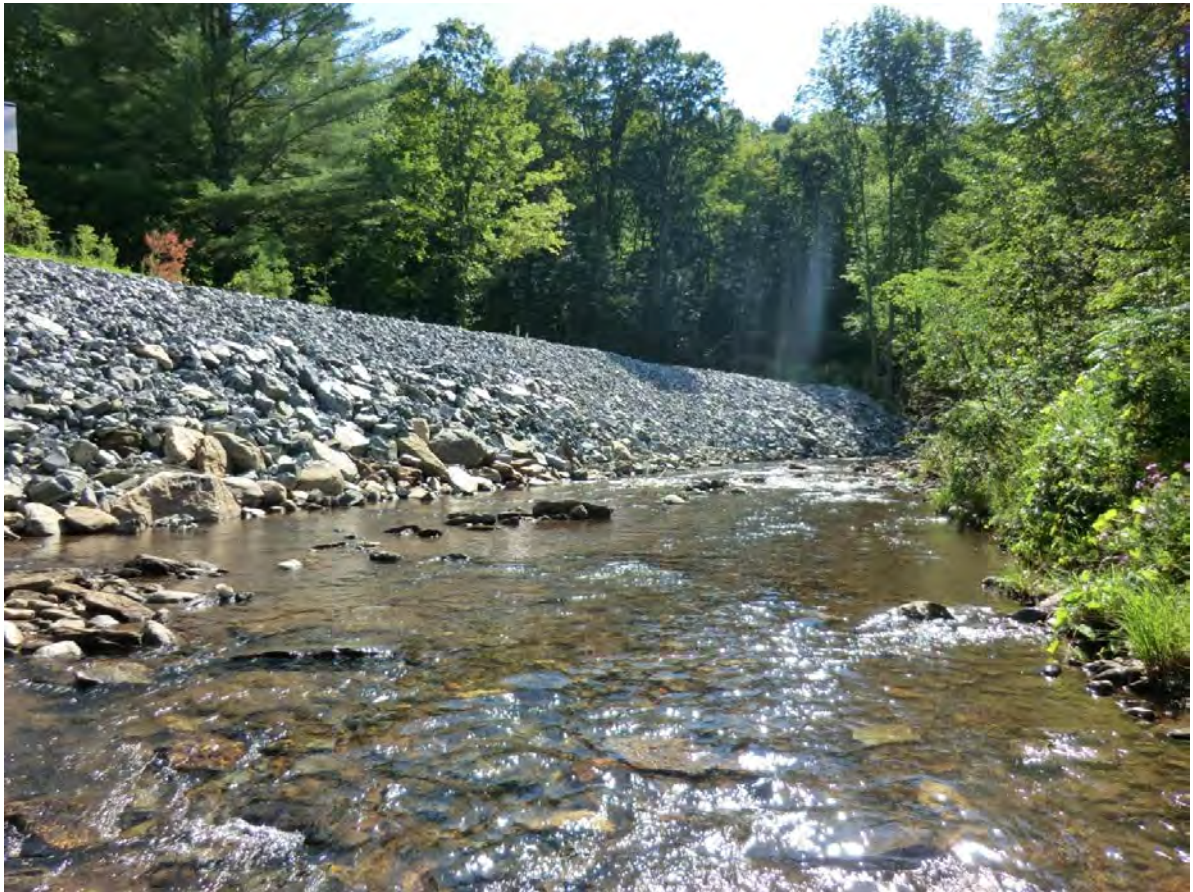
Figure 5.43. Extensive riprap above Route 4 bridge crossing.
