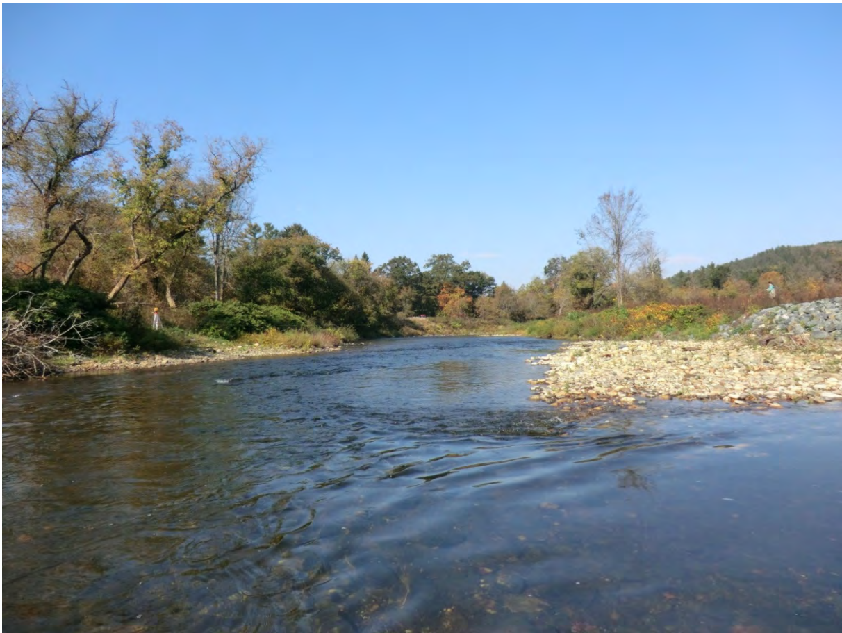
Figure 5.5. Widening and aggradation are occurring in M14-A. Rip rap prevents planform adjustment.
