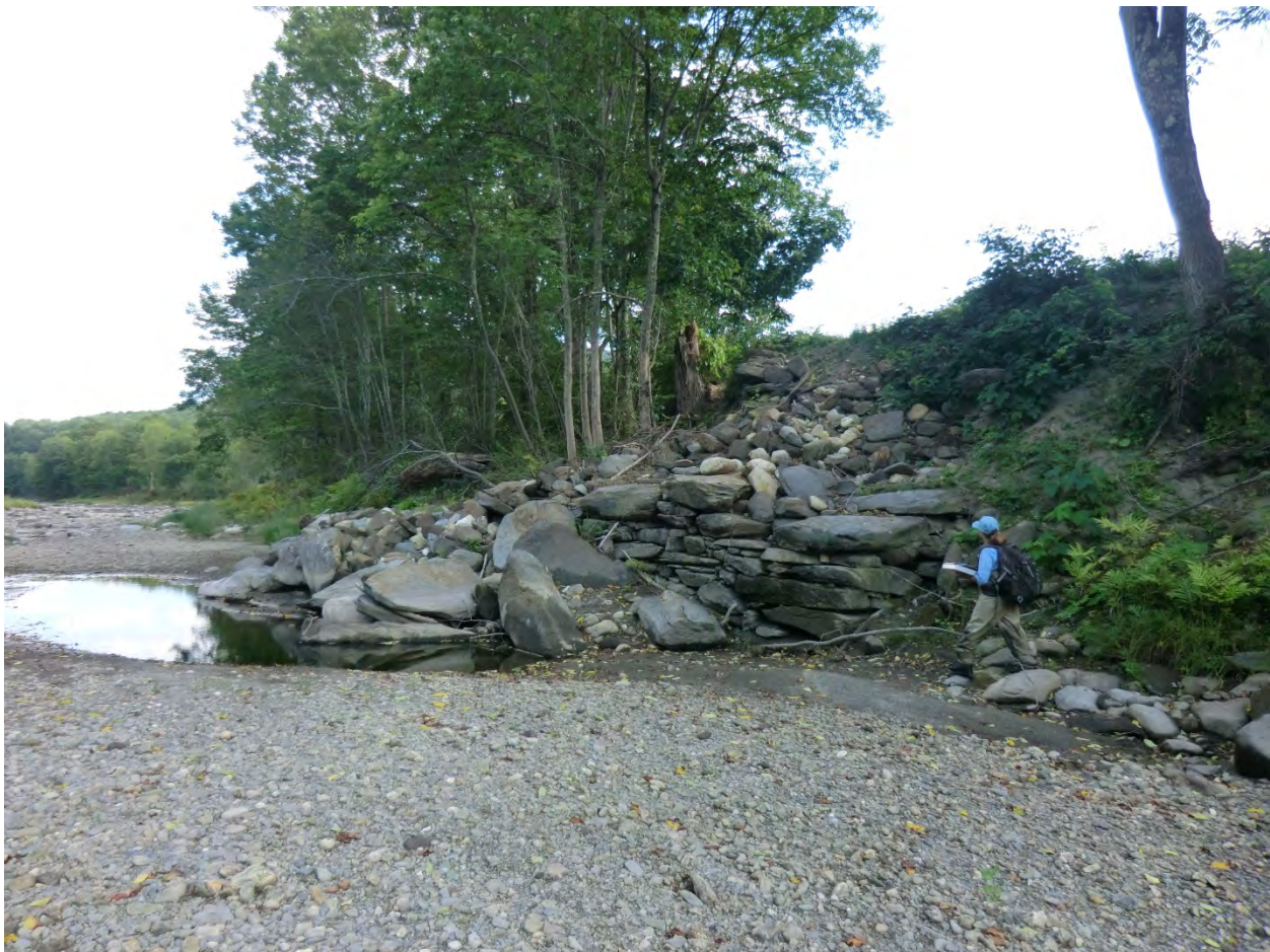
Figure 5.17. Old bridge abutment causing deposition in M21-A.
