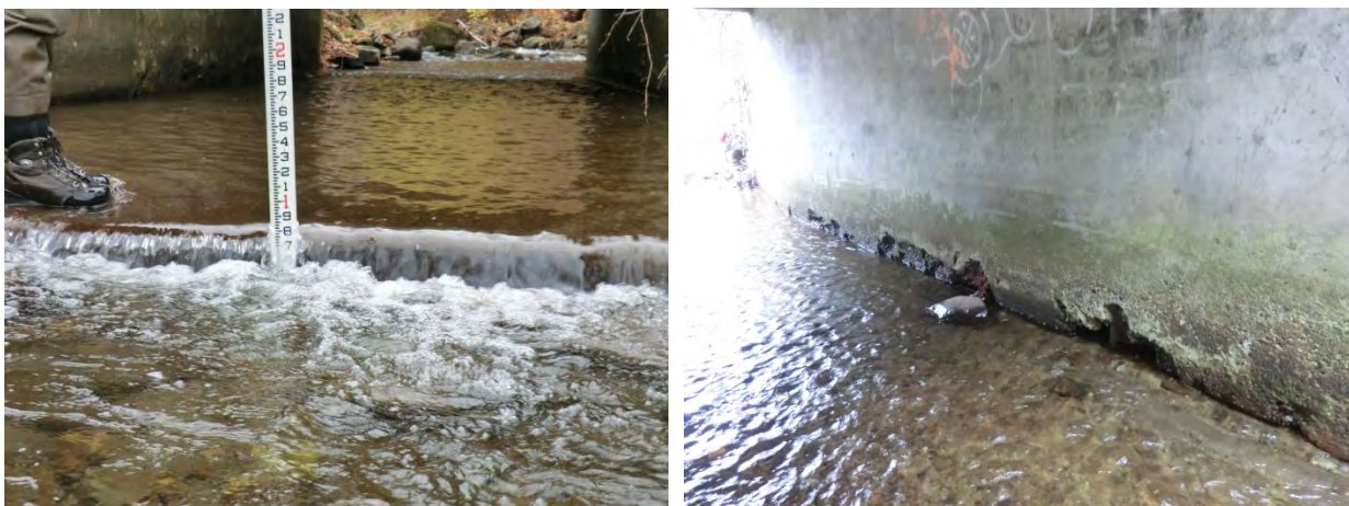
Figure 5.55. The most downstream box culvert on Avery Brook is perched at the downstream end and is deteriorating along the walls inside the structure.
