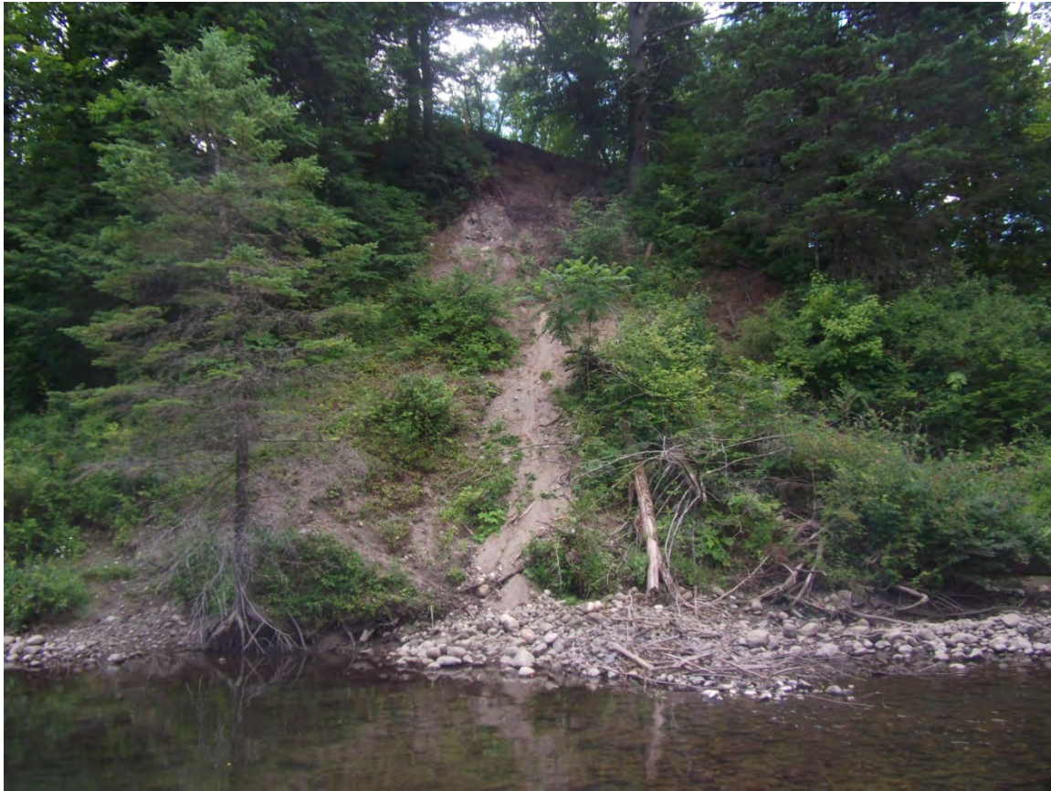
Figure 5.23. Mass failure on the bank in R11-A.
