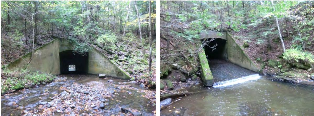
Figure 5.54. The Route 132 box culvert on Avery Brook limits aquatic organism passage.
