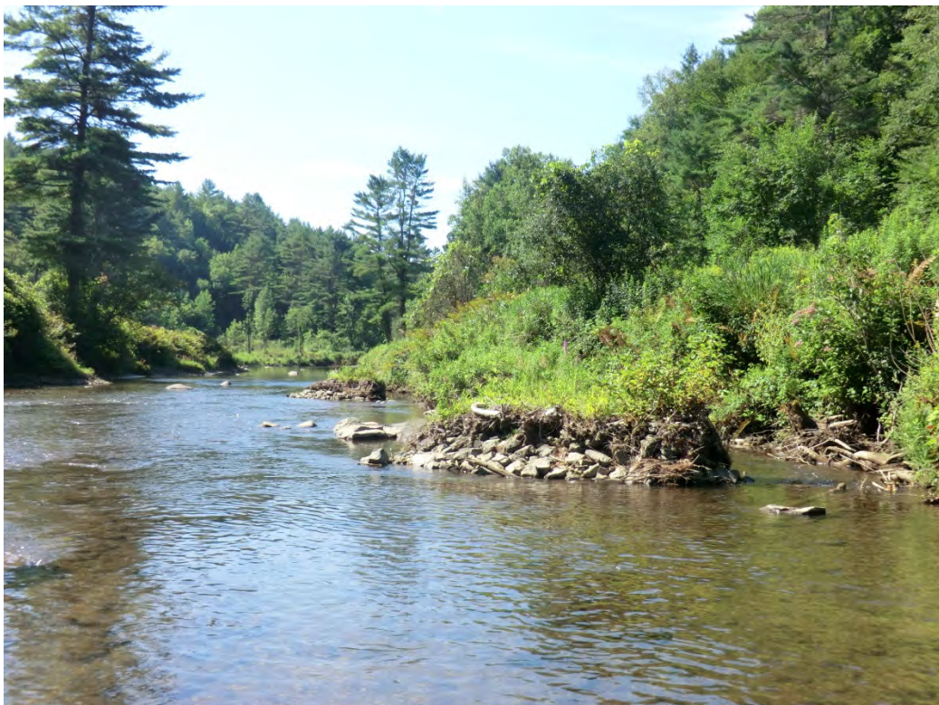
Figure 5.15. In some areas the river has outflanked the gabions and the channel flows on either side of them.
