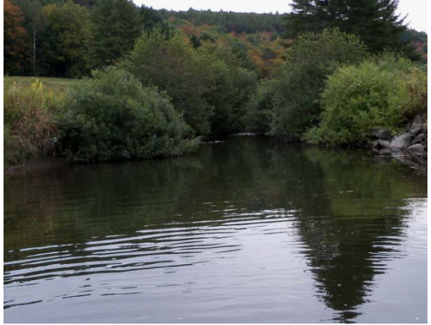
Scour below culvert
