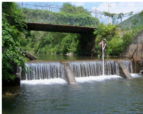
Figure 4.15 Geer dam in segment R19-B
