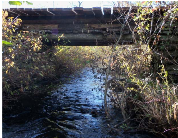
Project #4- Replace undersized bridge
