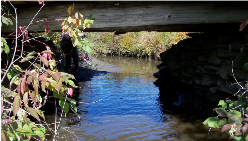
Project #5- Replace undersized bridge
