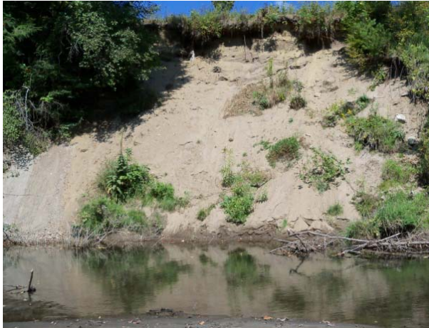
Project #7 – Improve stability of mass failure
