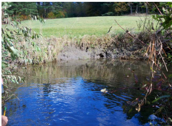
Figure 4.53 Lack of buffer and bank erosion
