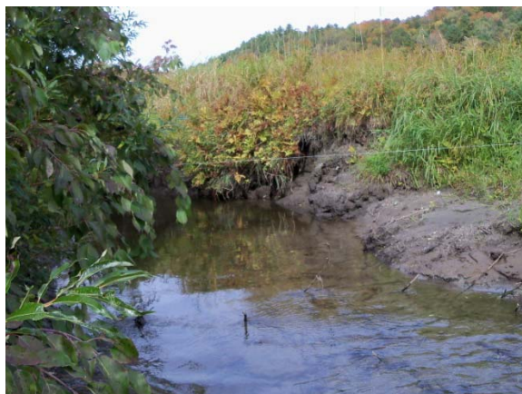
Figure 4.59 Bank slumping and typical channel
