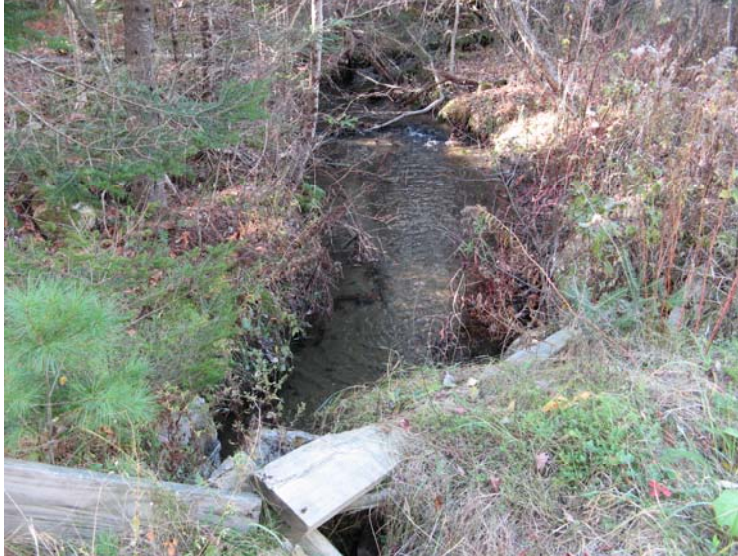
Figure 3 – Beaver Meadow Brook, approaching undersized culvert
