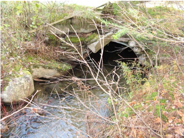
Figure 4 – Inlet to culvert with 25% bankfull width on Beaver Meadow Brook
