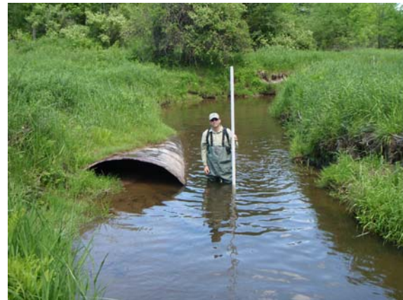
Figure 34 Failed old farm crossing in lower M11-A.
