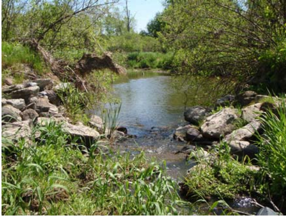
Figure 29. Old bridge abutment that has failed.
