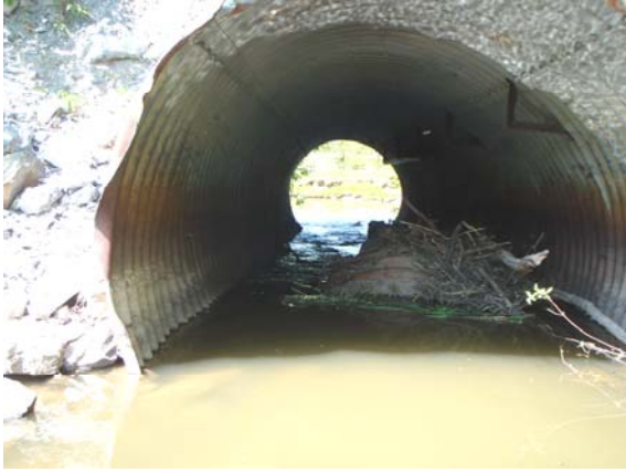
Figure 27. Debris jam inside the undersized culvert
