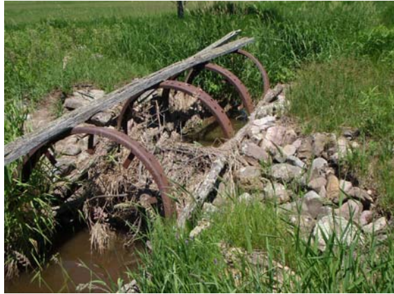
Figure 41. Culvert channel crossing clogged with debris
