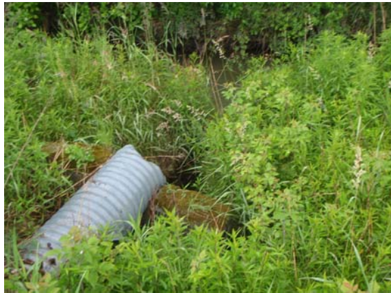
Figure 45. Interstate drainage eroding around a culvert
