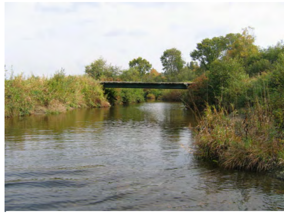
Figure 7.26. Farm bridge in T14-B with a span of 25 feet and a clearance of 5 feet.
