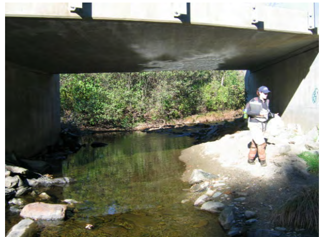
Figure 5.8 Large side bar within and downstream of Collinsville Road upper stream crossing. The alignment of the structure is poor and is causing localized geomorphic instability.
