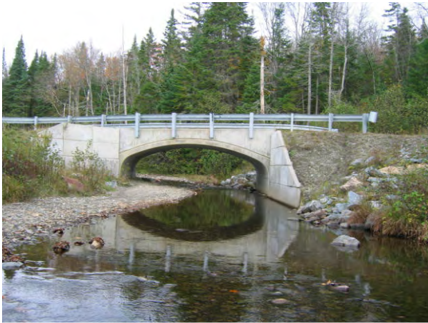
Figure 5.9 Deposition and scour above and below the Square Road Bridge. The bridge has poor alignment.
