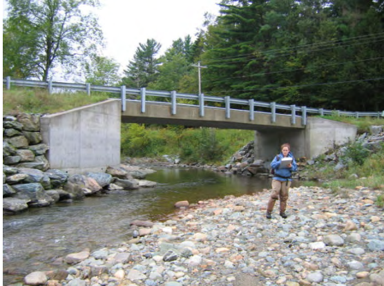
Figure 7.11. Sediment deposition upstream Tamarack Road Bridge. The bridge is undersized relative to the bankfull channel width and has poor alignment.
