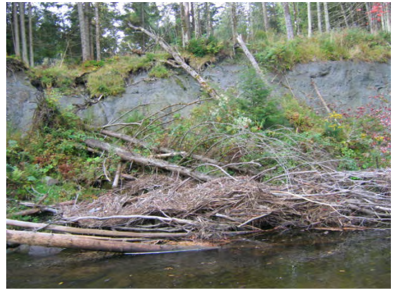
Figure 7.22. Debris jam in front of clay, east bank of T12-B. Mass failures as shown in this photo were common along the east bank.
