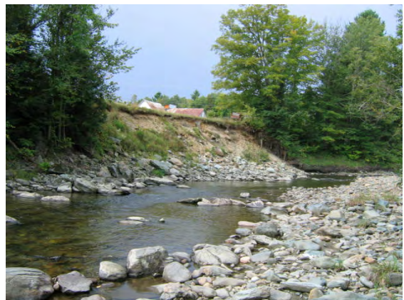
Figure 7.7. A mass failure about 15 feet high is on west bank where the Wild Branch flows away from North Wolcott Road in reach T04.
