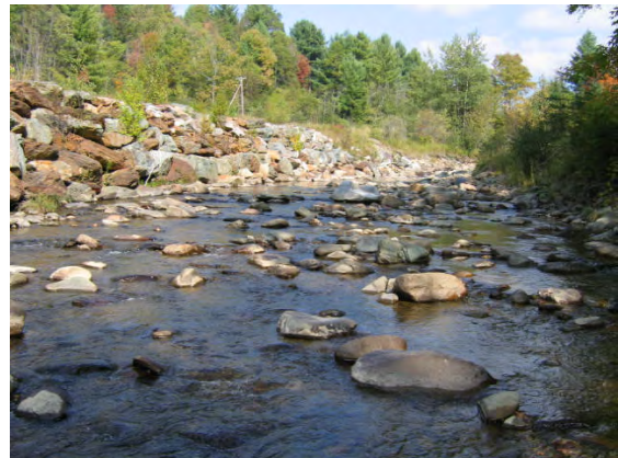
Figure 7.14. Segment T10-A has been extensively straightened and riprapped along the entire length.
