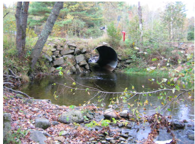
Figure 5.10 This undersized Brook Road stream crossing on a tributary to the Wild Branch is causing significant sediment transport problems as well as reduced aquatic organism passage.
