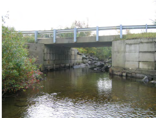
Figure 5.6 The Hatch Brook Road Bridge is undersized relative to the bankfull channel width.
