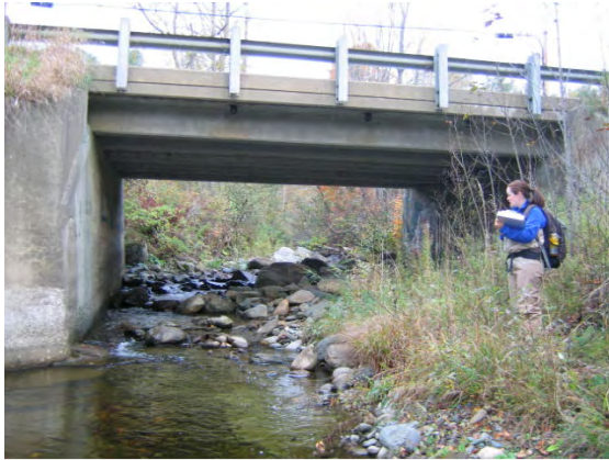
Figure 7.43. Deposition is occurring both upstream and downstream of the North Wolcott Road Bridge. This structure is a moderate priority for replacement.
