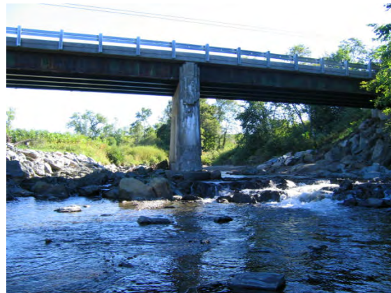
Figure 7.2. Downstream end of Route 15 Bridge showing deposition and ledge grade control within Reach T01
