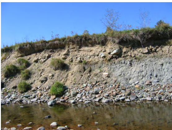
Figure 7.19. A mass failure approximately 15 feet high and 150 feet wide is located along the west bank of reach TII.
