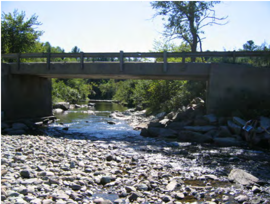
Figure 7.4. Rip rap and hard bank armoring is associated with the Gulf Road Bridge in Reach T03. The bridge is resulting in deposition of sediment.
