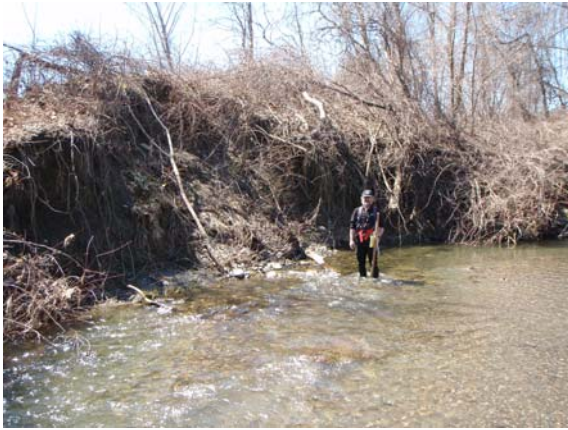
Figure 14. Mass failure in lower M01-B
