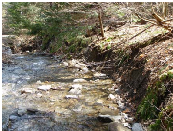
Figure 37. Bank erosion in lower T1.02-B.
