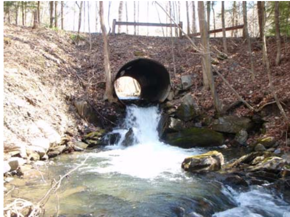
Figure 20. Perched culvert beneath Ryan Road.
