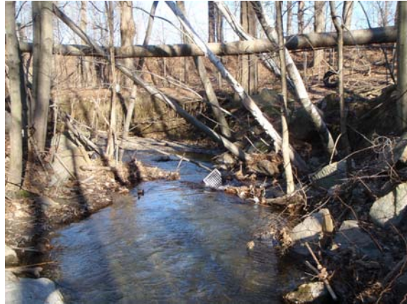
Figure 32. Severe bank erosion below I-91 culvert.
