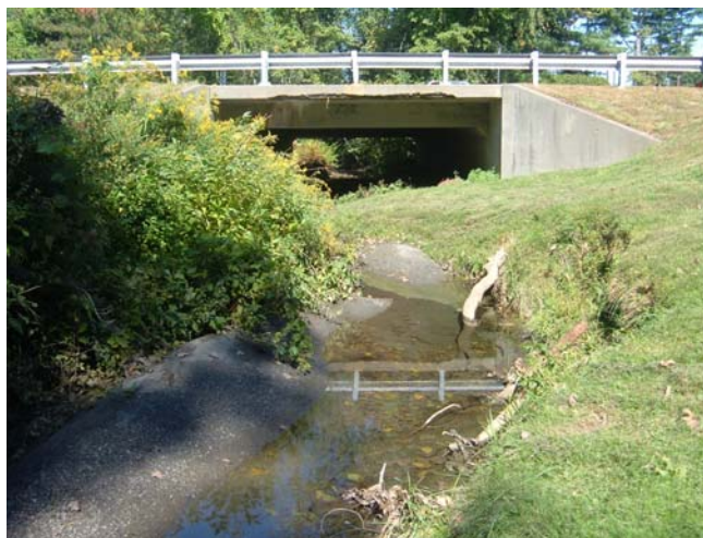
Figure 7. Depositional features below the I-91 Exit 3 box culvert.
