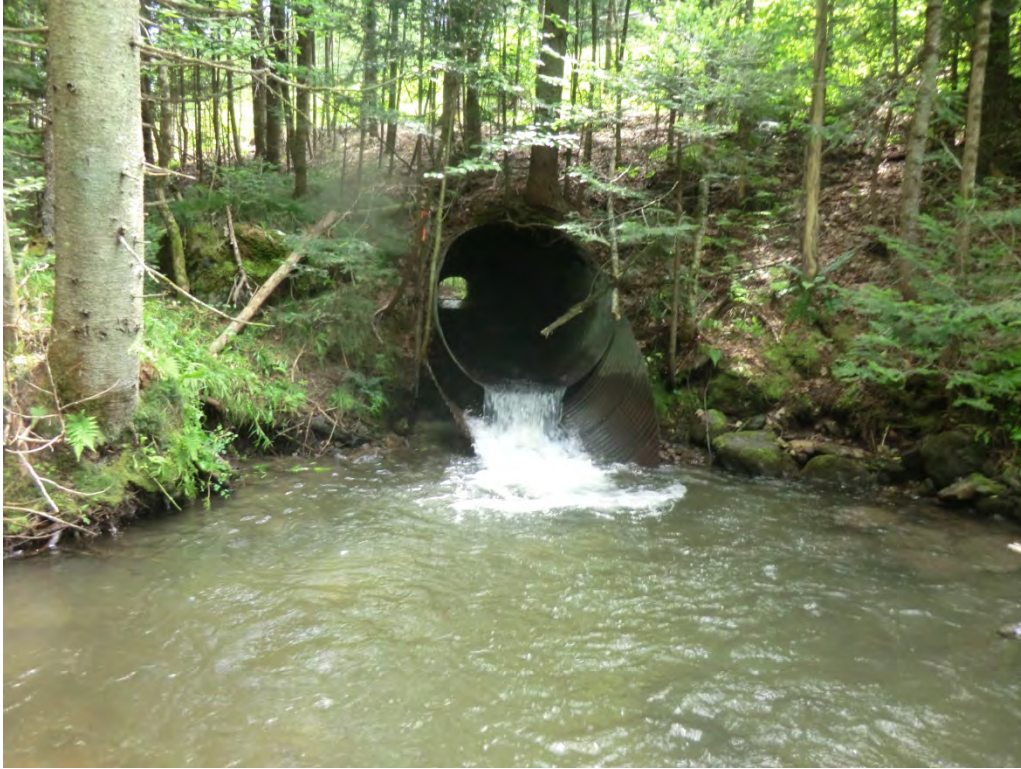
Figure 5.30. Undersized culvert causing potential fish passage issue with culvert apron falling off in T1.01.
