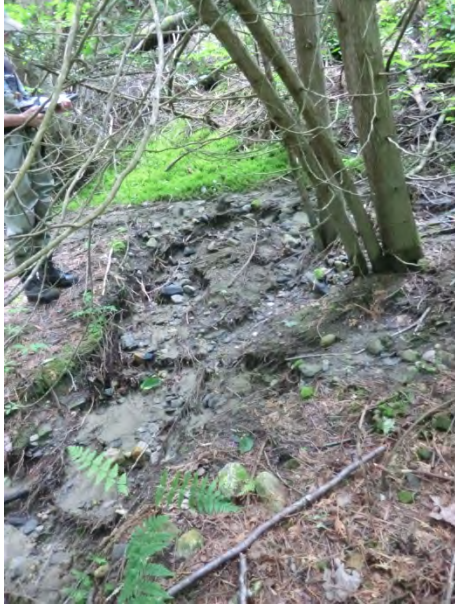
Overland stormwater runoff in T1.01
