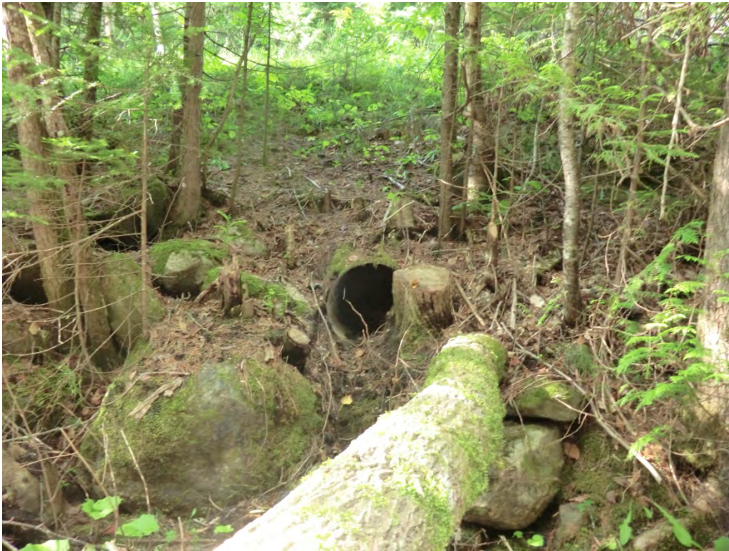
Figure 5.13. Stormwater drainage pipe contributing sediment to Dishmill Brook in M103.
