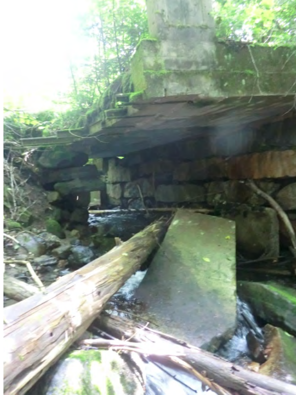
Figure 5.32. Bridge failure at trail crossing in T1.01.
