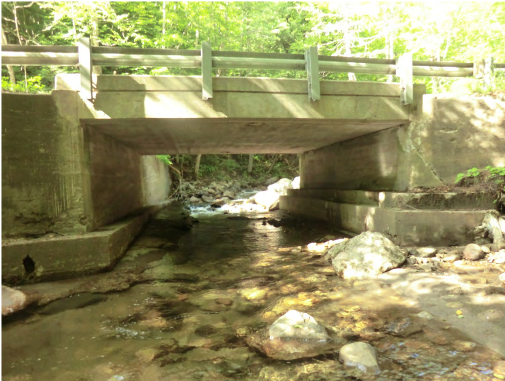
Figure 5.29. Undersized structure at Mountain Road crossing causing geomorphic instability in M103.
