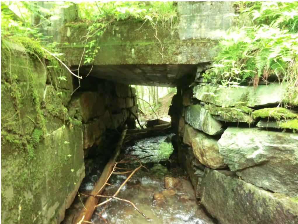
Figure 5.31. Channel constriction at trail crossing in reach T1.01.
