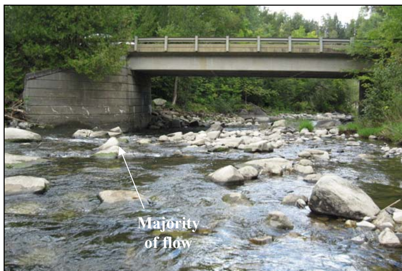
Figure 9: Example of sediment deposition upstream of bridge on Willoughby River Reach T3.
