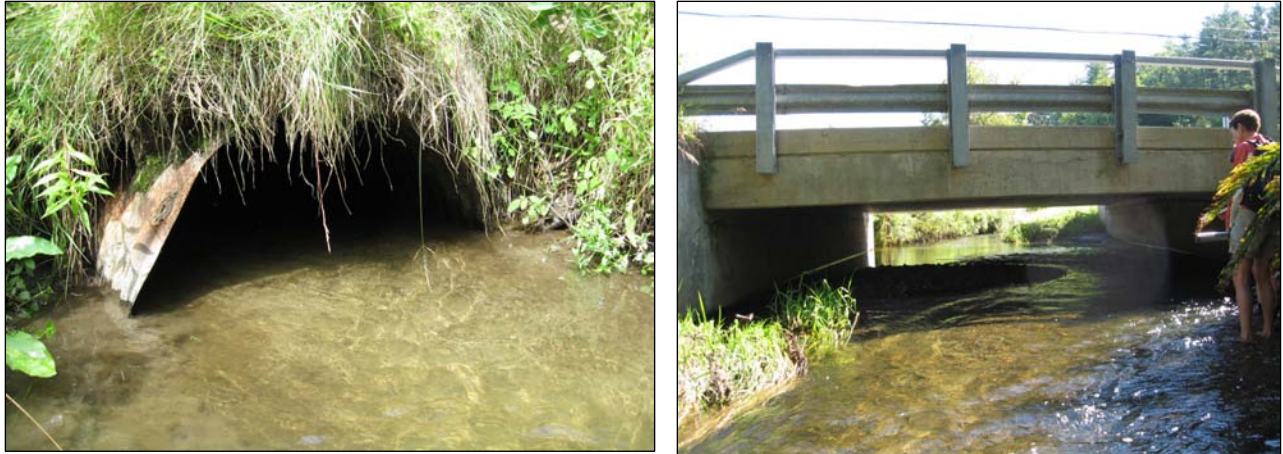
Figure 43: Sediment accumulation downstream of culvert on Reach T1.01; deposition beneath bridge on M05.
