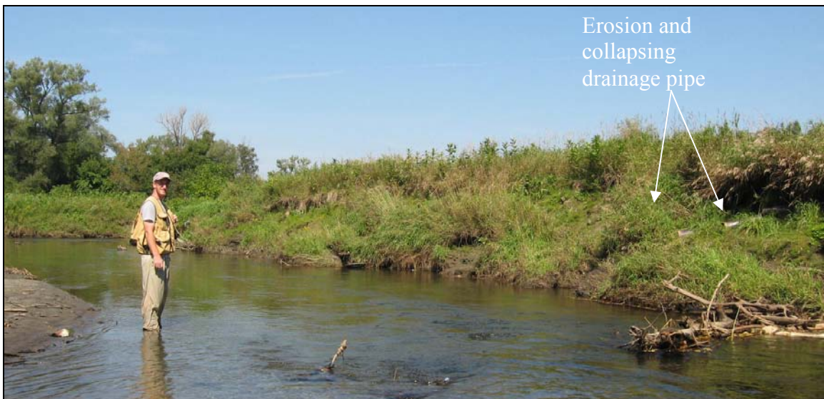
Figure 28: Extensive erosion in this area of Reach M08 has caused several sections of a drainage pipe to collapse.
