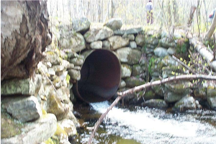
Figure 4. Undersized culvert located in Reach M05.
