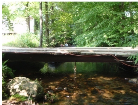
Figure 4.60 Bridge with low clearance; 22 ft construction
