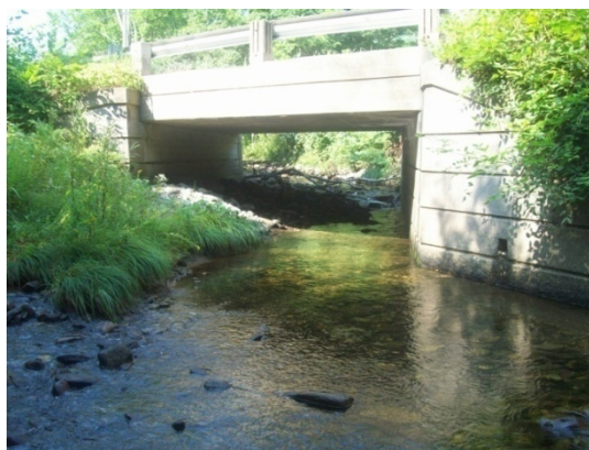
Figure 4.79 Sediment deposition within undersized bridge
