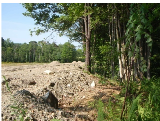
Figure 4.57 Exposed surficial material with no sediment BMPs
