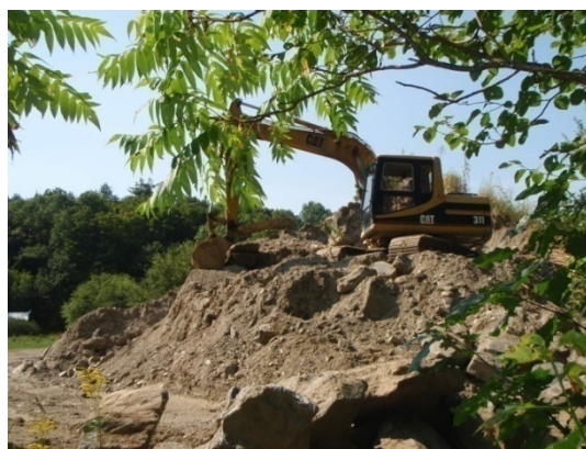
Figure 4.58 Fill and excavator within 25 feet of channel
