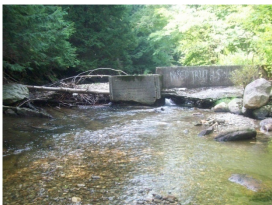
Figure 4.68 Breached dam upstream of Kidder Hill Road
