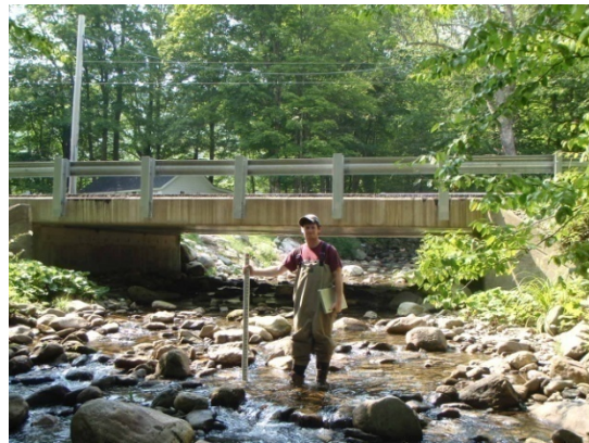
Figure 4.89 Undersized crossing at Townshend Road
