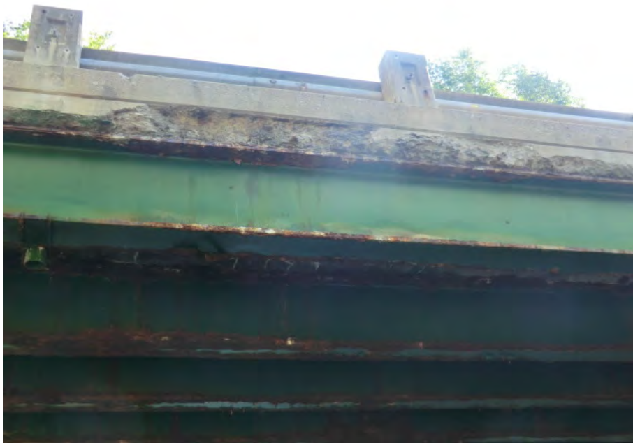
Figure 5.20. Deteriorating decking and rusting beams of Rt. 100 bridge in segment T8.05-C.
