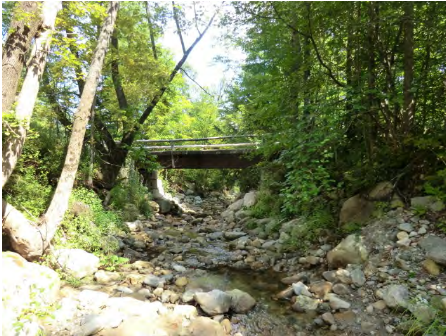
Figure 5.23. Private driveway bridge in T8.S3.01 recommended for replacement.
