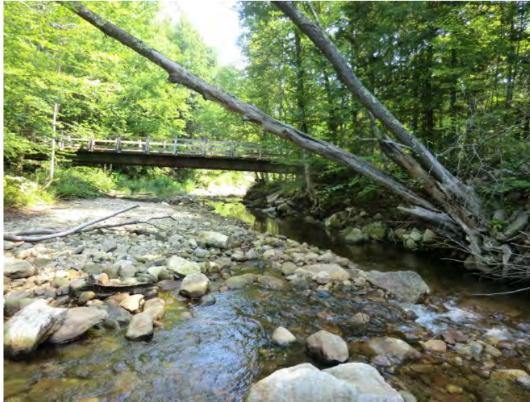
Figure 5.21. Temple Road bridge in segment T8.06-B recommended for replacement.
