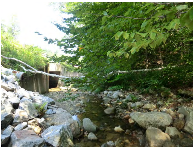
Figure 5.22. Poor alignment of Dover Brook culvert under Rt. 100 and Cross Rd.
