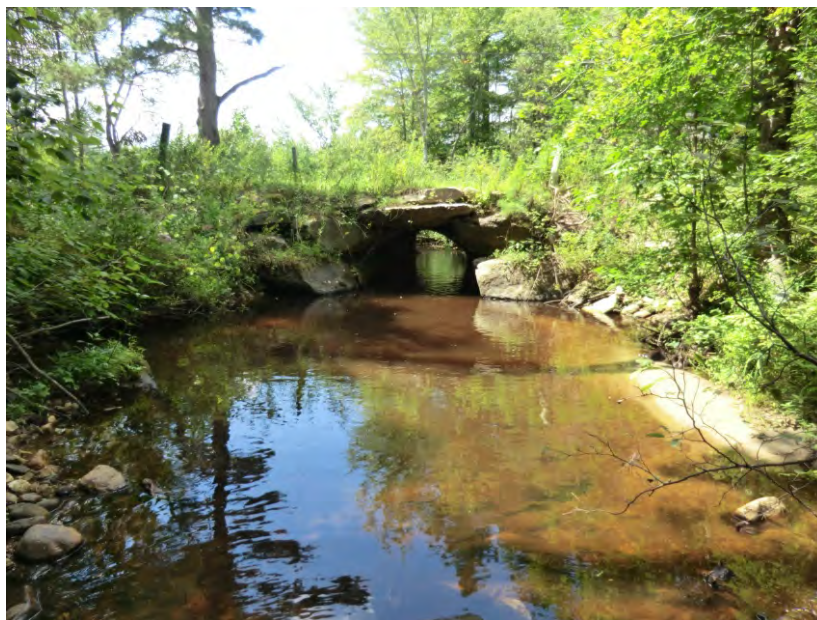
Figure 5.33. A culvert under River Road in T11.S3.01-A is very undersized.
