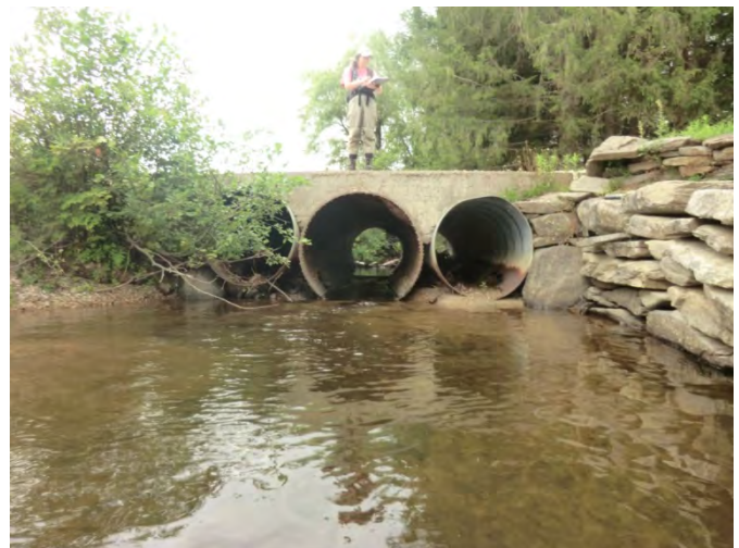
Figure 5.38. One of three culverts under Stratton View Rd in T11.S4.01-B is rusted out.
