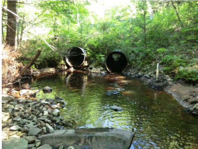
Figure 5.34. One culvert captures all baseflow and the other is rusting out at Raspberry Hill in T11.S3.01-B.
