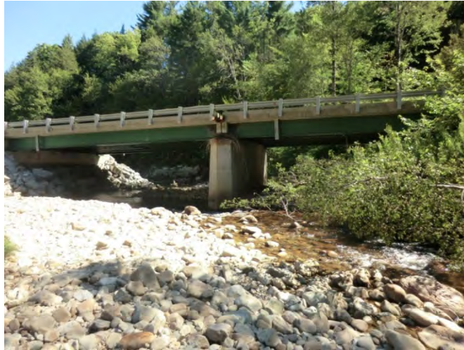
Figure 5.30. Rt. 30 bridge with aggradation and alignment problems in T11.04.
