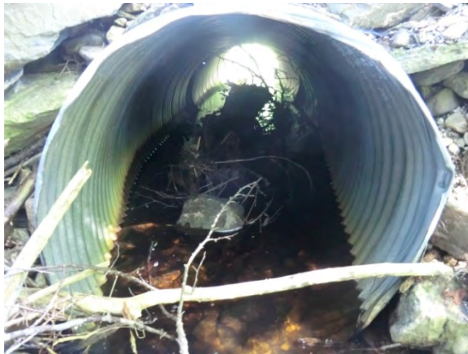
Figure 5.35. The culvert on Red Brook under Cranberry Hill Rd is full of woody debris.
