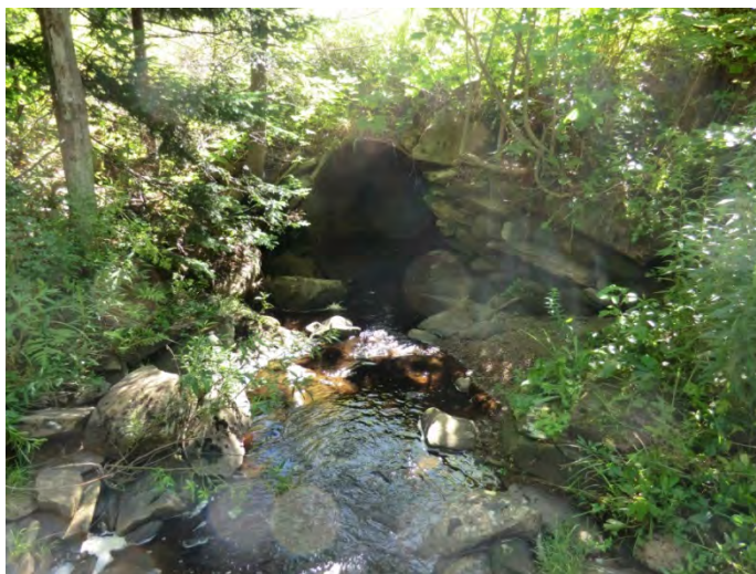
Figure 5.36. The culvert under Winhall Hollow Rd is not well aligned.
