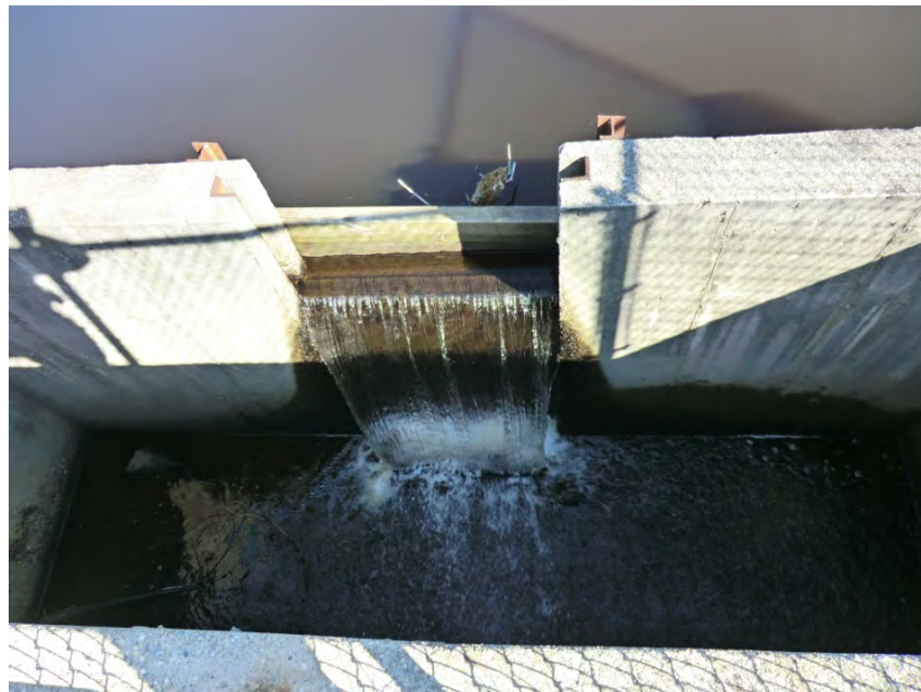
Figure 5.22. The dam at the pond outlet likely poses an AOP barrier.
