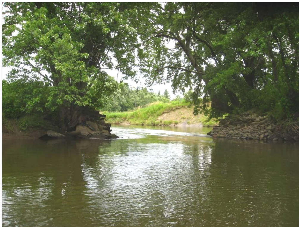
Figure 11: Old abutment on Reach M16. Note narrow constriction, upstream scour pool, and resulting erosion downstream.
