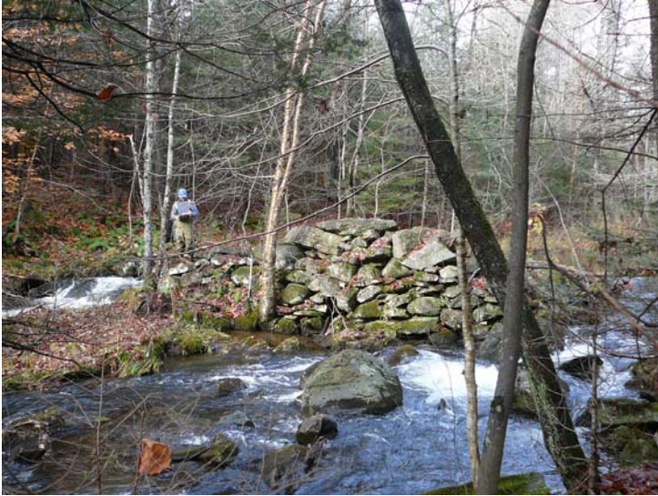
Figure 10. Remnants of breached dam at bifurcation in Patch Brook channel. View upstream, M40T5.03 Segment B, Patch Brook; 29 October 2009
