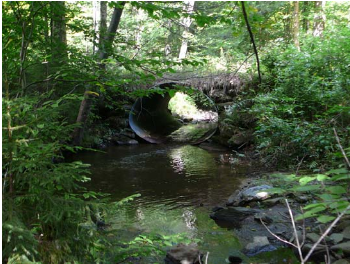
Figure 29. View upstream, to bankfull constricting culvert crossing under Reading Pond Road, Segment B, M41T6.02S1.02, Reading Pond Brook, 4 September 2009.
