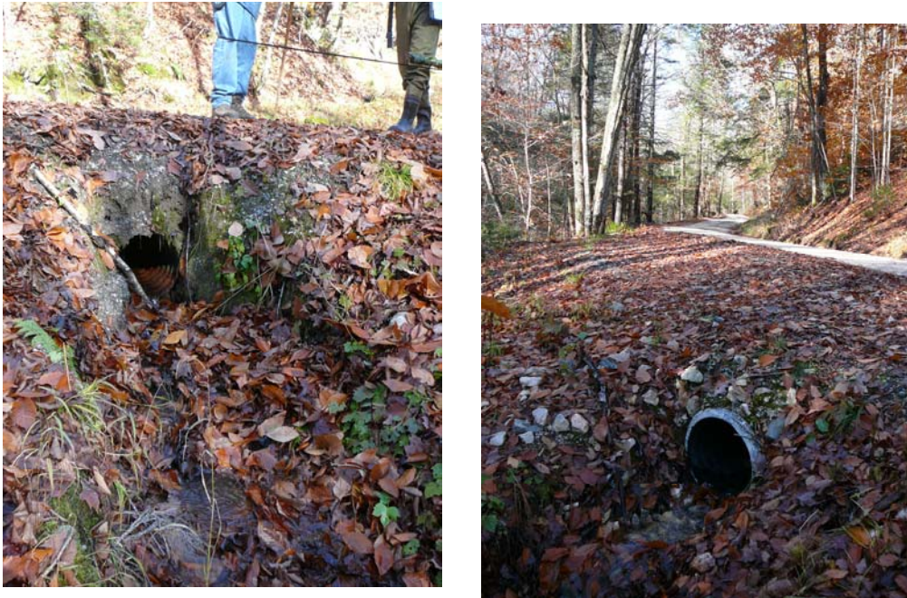
Figure 9. Stormwater inputs to Patch Brook, M40T5.03 Segment B, from Patch Brook Road; 29 October 2009. (a) cross culverts without headers are sites of road sediment runoff to the channel; (b) sections of the road are graded to drain directly to the channel.
