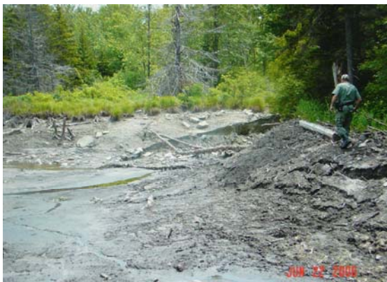
(c) breached dam, 22 June 2006 (Source: VTDEC).
