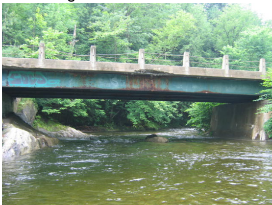
Figure 7.41. Bridge crossing of Nebraska Valley Road constricting Reach T4.02
