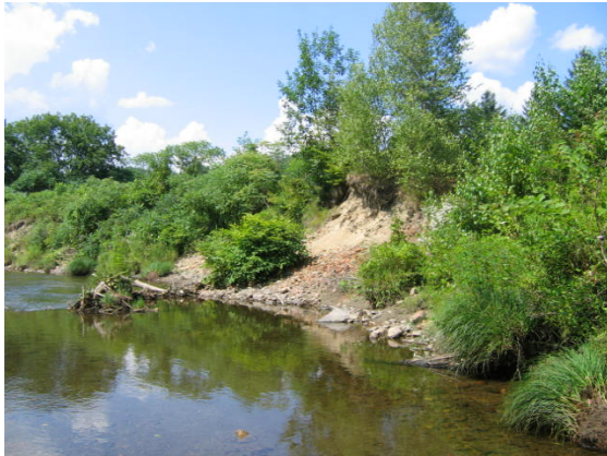
Figure 7.7. Bank erosion along M09
