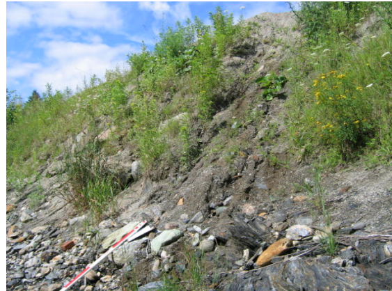
Figure 7.23. Bank erosion and lack of woody vegetation in the vicinity of the municipal sand storage facility
