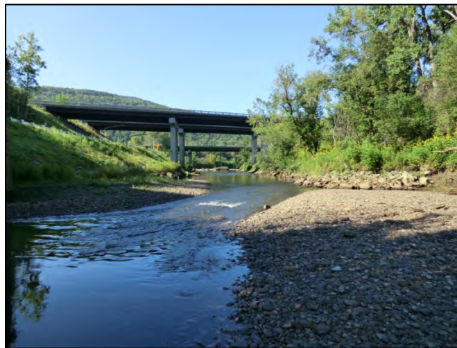
Figure 5.12. M2.01 impacted by valley width changes by placement of I 89 and Route 2 bridges.
