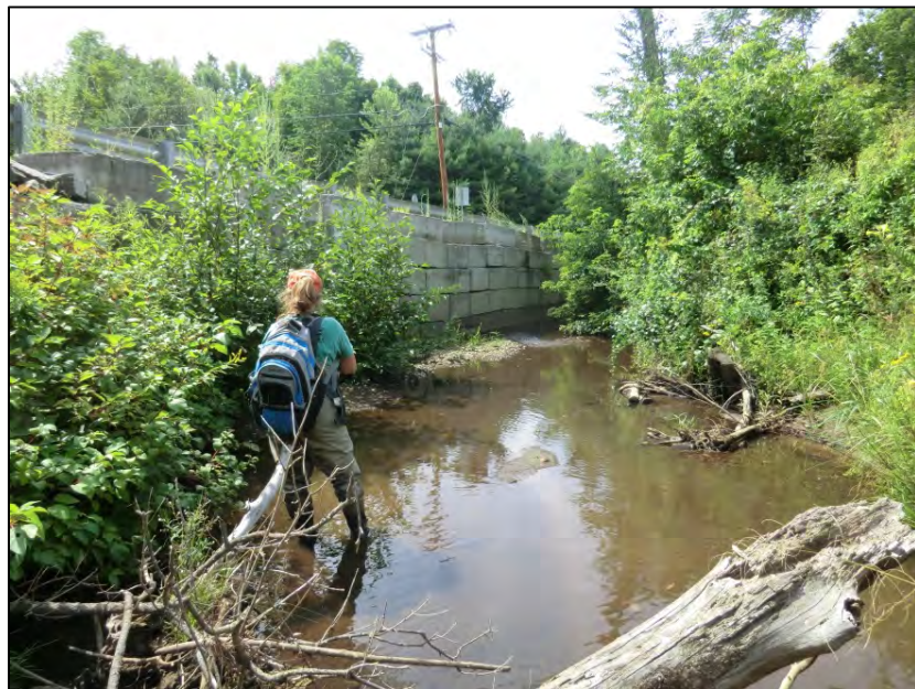
Figure 5.22. Concrete block wall against Lincoln Street armoring the stream bank along Graves Brook.
