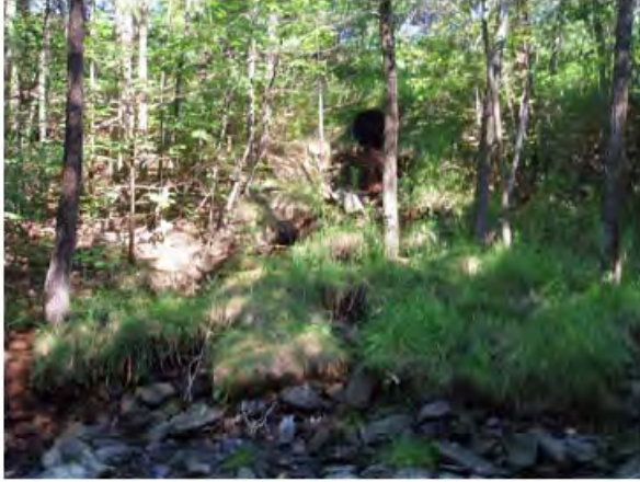
Figure 2: Deer Brook M02- Stormwater Input
