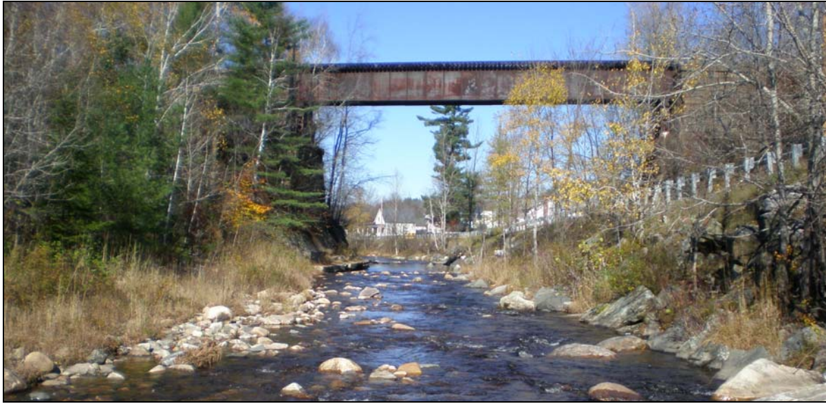
Figure 33: The railroad bridge span on M11-A is adequate for the Mill River, however, location of Route 155 in relation to the bridge and the river creates a channel constriction between the bridge abutment and the road.
