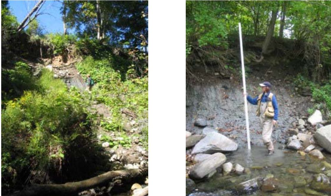
Figure 9. Mass failure in M05A (left) and bank failure in M05B (right) are indicative of channel adjustment processes in Reach M05.
