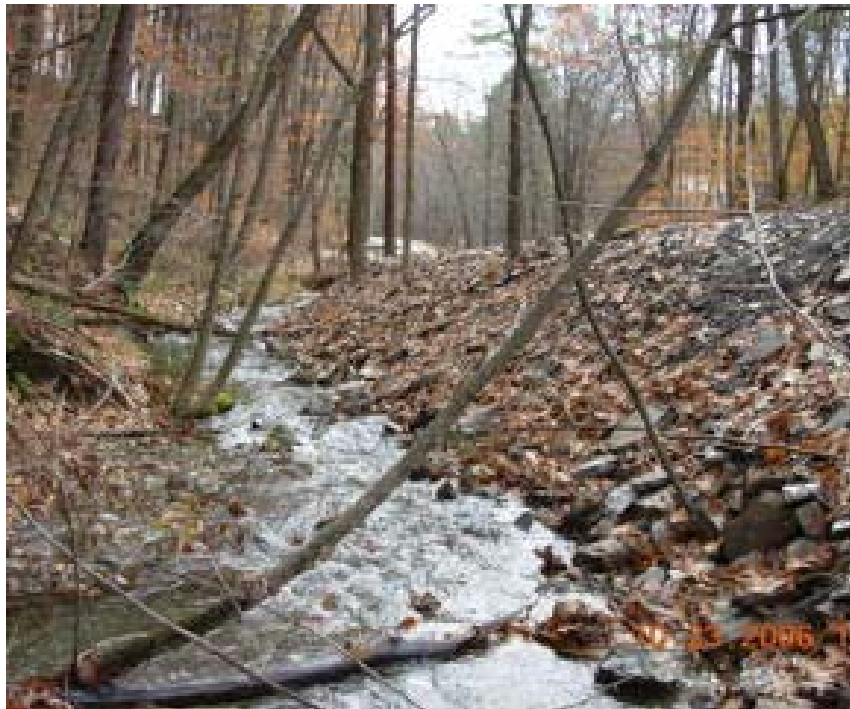
Figure 28. M03-T1.03A, similar to many of the reaches assessed in the Phase 2 study of the Blood Brook watershed, was characterized by human development and frequent road encroachment.
