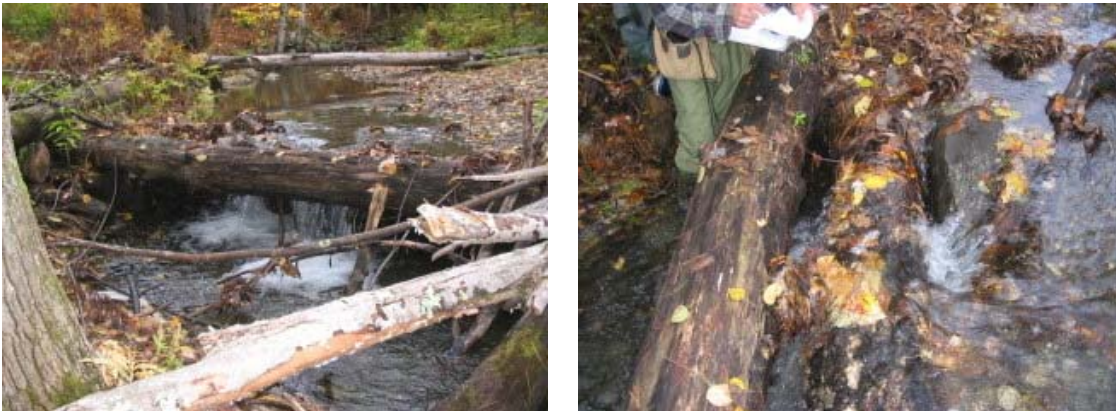
Figure 18. A log dam in segment M08-C (left) that appears to have been installed as part of a stream ford to access a log landing has been eroded and is now forming an active headcut with the potential to migrate upstream rapidly (right).
