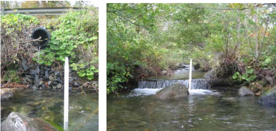
Figure 16. An elevated pipe carrying overflow from a pond above the floodplain daylights on the steep banks below Turnpike Rd. in segment M08-A (left). Degradation of erodible bed materials below this outfall has formed a 3 ft. deep pool, and concern about upstream migration of this downcutting may be a primary reason for installation of a check dam just upstream of this point (right).
