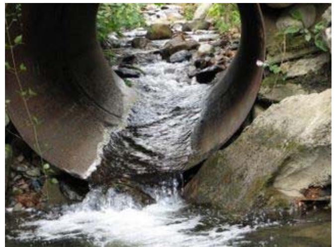
Figure 19. Indications of scour undermining this culvert make the possibility of upstream migration of headcuts a concern for structural integrity. Sediment deposition above, not as heavy at this culvert as some others in the study, indicates a structure may not be adequately sized to transport sediment as well as water at bankfull flows.
