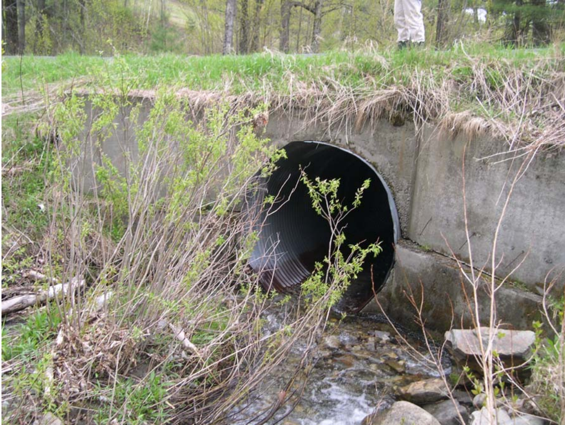
Figure 6 – Sediment Transport Impeded at Old Orchard Lane on mainstem
