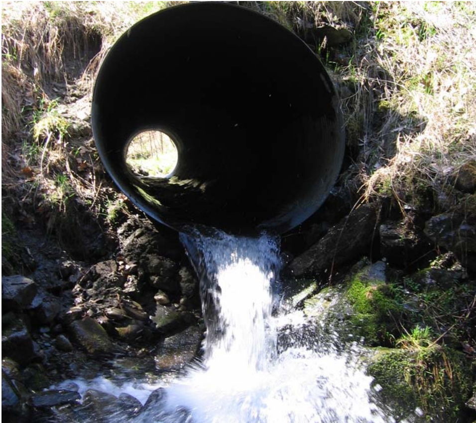
Figure 4 – Perched Outlet Poor Installation on Bragg Hill Road
