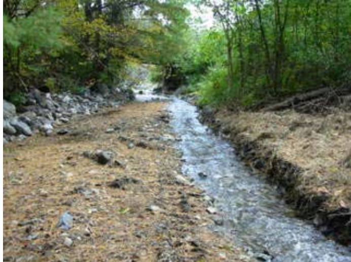
Figure 34. Recent dredging just upstream of a private bridge replacement project in Reach M06.
