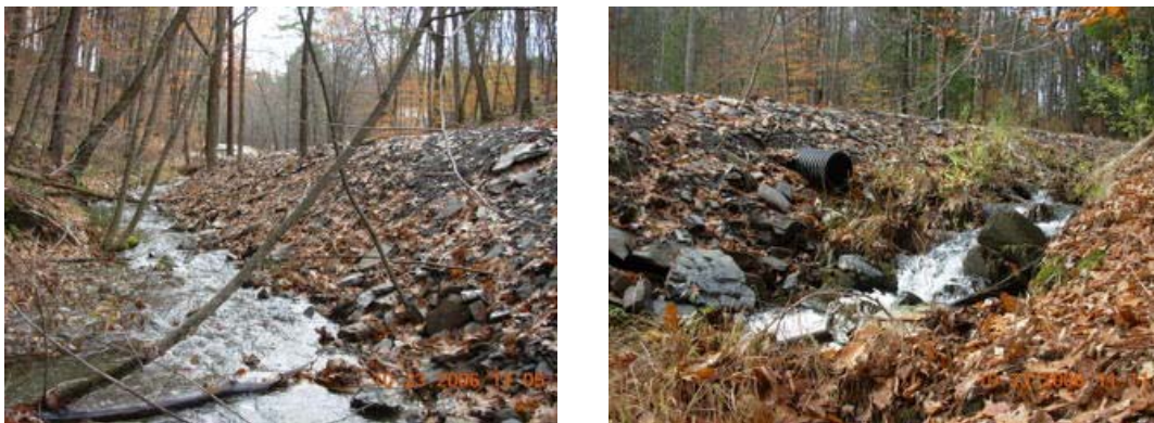
Figure 57. Encroachments along more than 20% of segment M03-T1.03A contribute to an increase in stream power.
