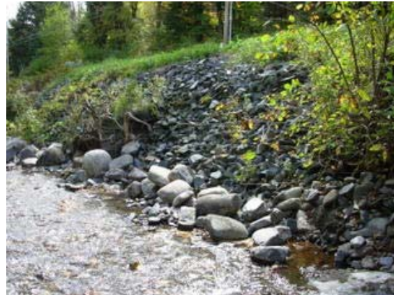
Figure 32. Road encroachment in reach M06 sometimes confines the stream sufficiently to change both the valley confinement type and stream type (C to B) over short distances.
