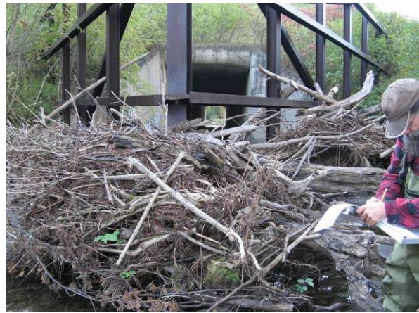
Figure 5. This debris catcher is located at the mouth of a 70-foot-long box culvert that runs underneath Rte. 5 at the downstream end of reach M03 on the Blood Brook mainstem, where floodwaters nearly overtopped the embankments in 1973 (Fig. 6).
