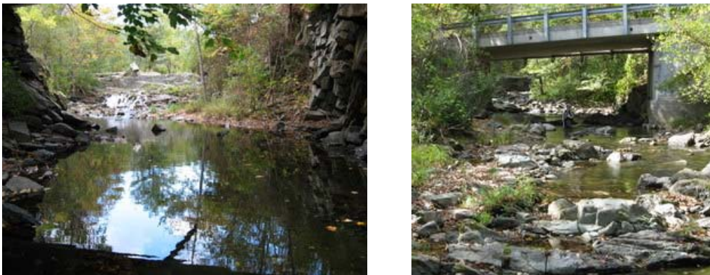
Figure 26. The bridges at Elm St. (left) and Hopson Rd. (right) were built near the locations of waterfalls. Substantial bedrock outcrops at these locations increase stream stability and limit channel adjustments but also create channel and floodplain obstructions that could increase the possibility of channel avulsion in a flood or ice jam.
