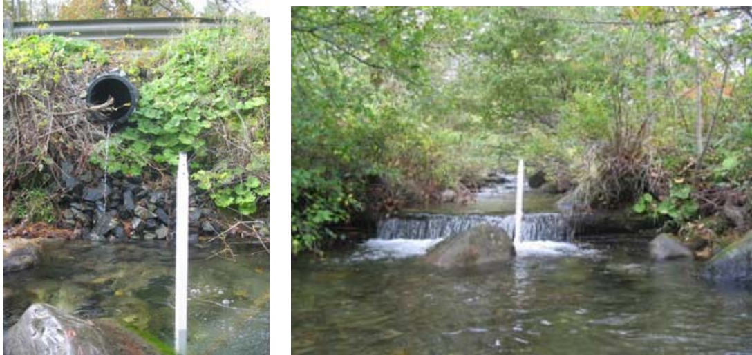
Figure 40. An elevated pipe carrying overflow from a pond above the floodplain daylights on the steep banks below Turnpike Rd. in segment M08A (left). Degradation of erodible bed materials below this outfall has formed a 3-foot-deep pool, and concern about upstream migration of this downcutting may be a primary reason for installation of a check dam just upstream of this point (right).
