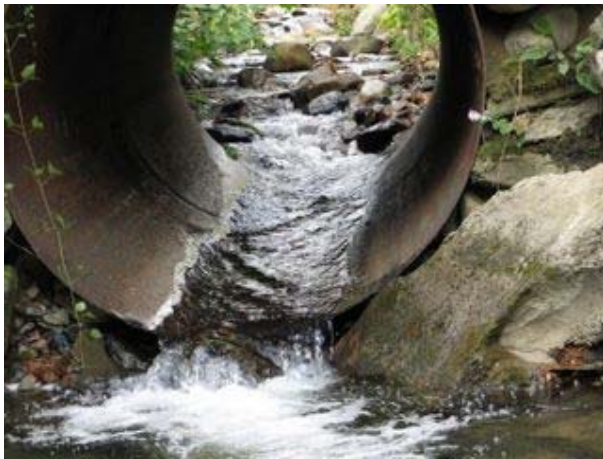
Figure 44. Indications of scour undermining this culvert make the possibility of upstream migration of headcuts a concern for structural integrity. Sediment deposition above – not as heavy at this culvert as some others in the study – indicates a structure may not be adequately sized to transport sediment as well as water at bankfull flows.
