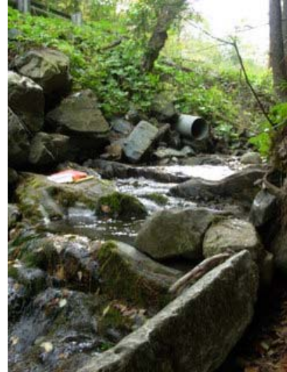
Figure 53. Road encroachment and channel constrictions such as this culvert in segment M03-T1.02B can combine to create localized increases in stream power and decreases in sediment load that increase the likelihood of downcutting processes.
