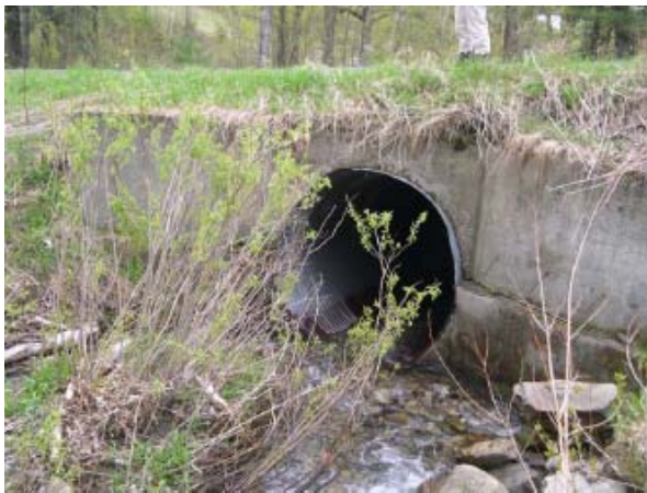
Figure 16. Cumulative deposition now obstructing a culvert at Old Orchard Ln. indicates the culvert is not sized adequately to transport sediment as well as water at high flows (photo courtesy of TRORC 2006).
